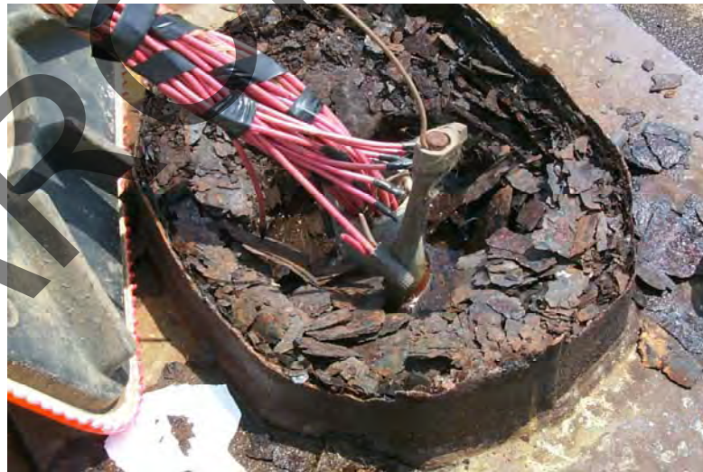
Figure 2. Failure of Weathering Steel Pole. Note the Corrosion Product.
