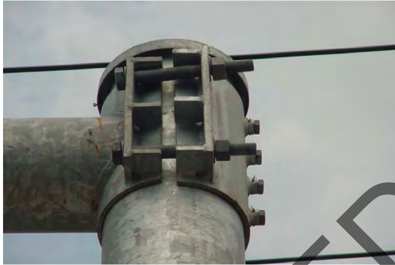
Figure 27. Post to Arm Connection Showing Poor Fit-Up Due to Use of Incorrect Components.
