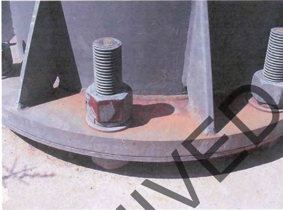
PHOTOGRAPH 5: LIGHT CORROSION ON BASE PLATE
