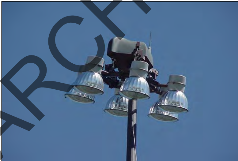
Figure 30. Misaligned Luminaire Ring.
