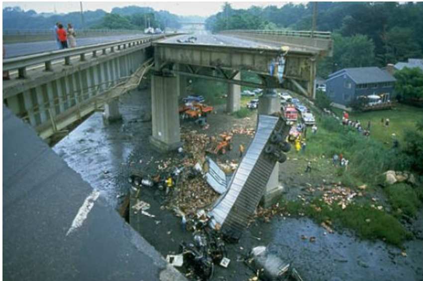
Figure 7.1-2 Collapse of the Mianus River Bridge.
