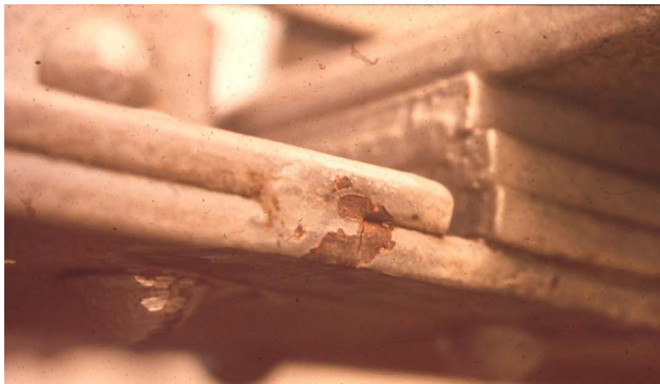
Figure 9.1.2-4 Fatigue crack at toe of tack weld.
