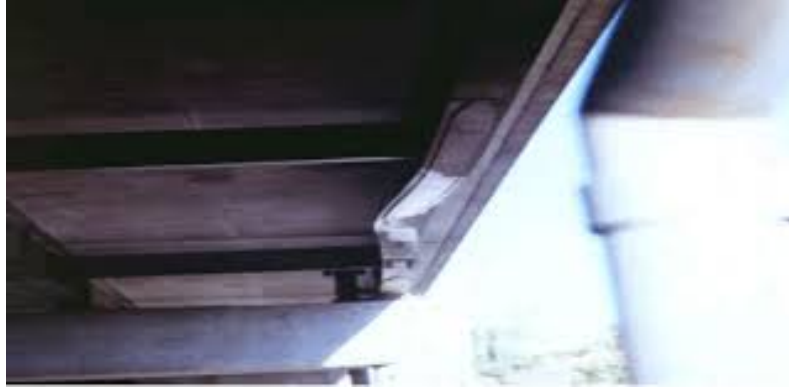
Figure 9.3.2-1 Damage to a steel bridge girder due to an over-height vehicle collision.
