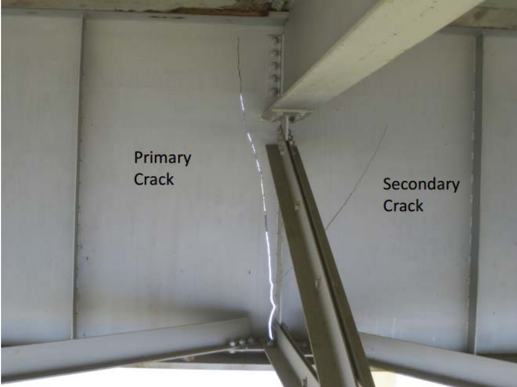
Figure 7.2.4.1-6 CIF cracks in the Diefenbaker Bridge.
