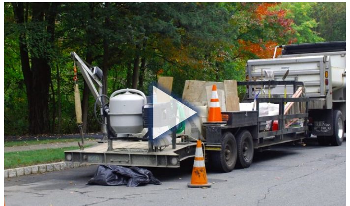
Watch a New Jersey DOT video to learn more about Montgomery Township's inlet repair trailer.
