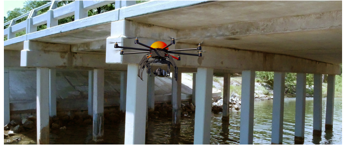
UAS can support traditional bridge inspection practices to provide rapid, high-quality data.
