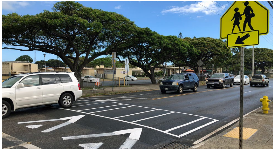
Hawaii DOT installed raised crosswalks on Kalihi Street in 2019, a section of roadway that had previously averaged two pedestrian-related crashes per year.
