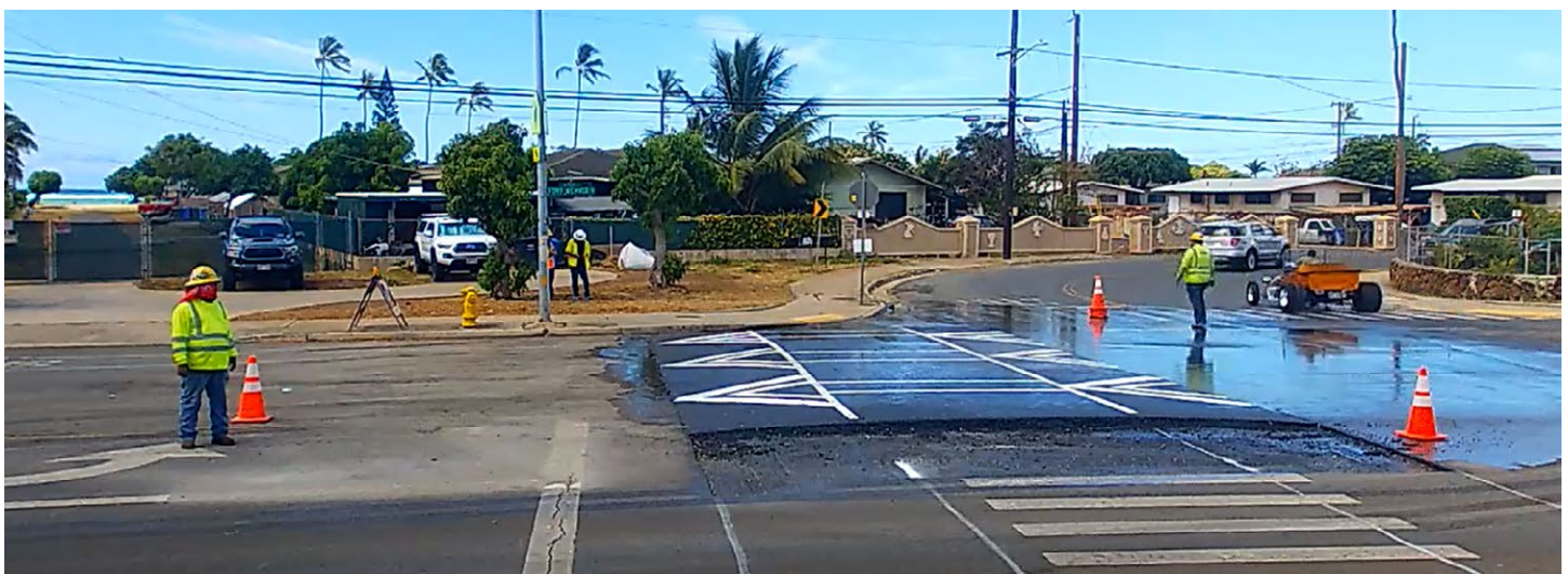
Raised crosswalks improve the visibility of pedestrians and provide drivers a physical reminder to reduce their speeds.
