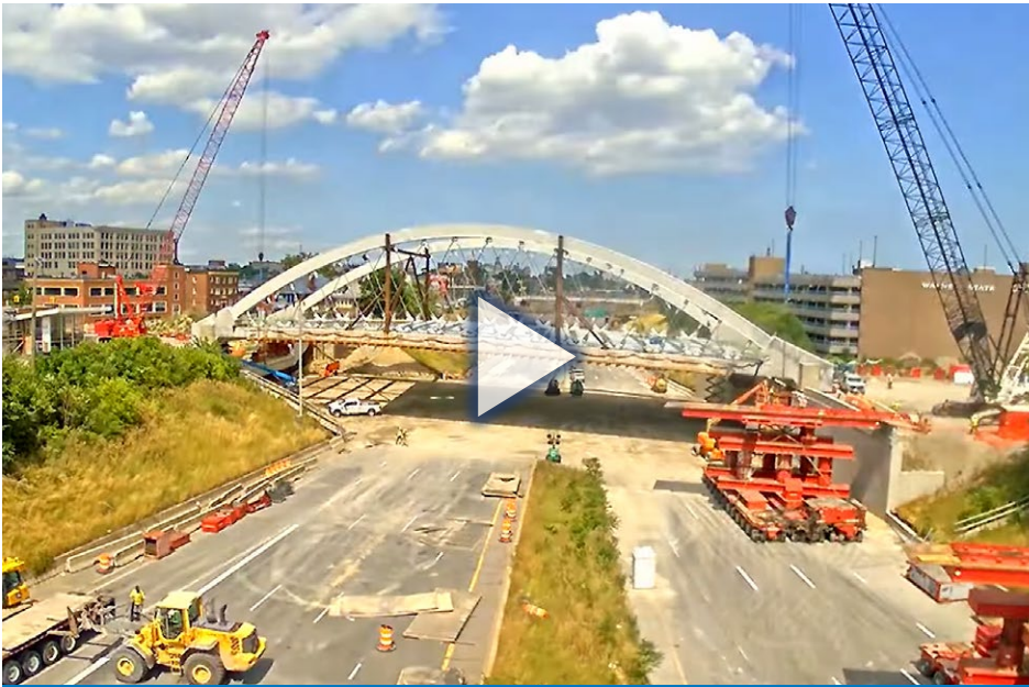
Watch a time-lapse video of Michigan DOT moving a new bridge over I-94 into place.
