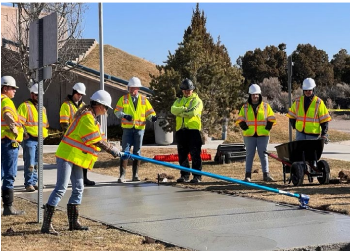
ICONIC training program students replaced a concrete sidewalk at an interstate rest area in partnership with Idaho Transportation Department staff.
