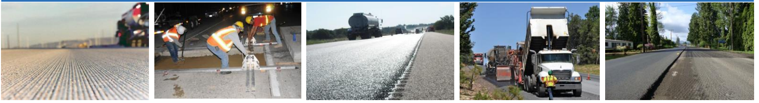
Photo sources: (1) American Concrete Pavement Association; (2) Utah DOT; (3) Applied Pavement Technology, Inc.; (4) National Park Service; (5) Washington State DOT
