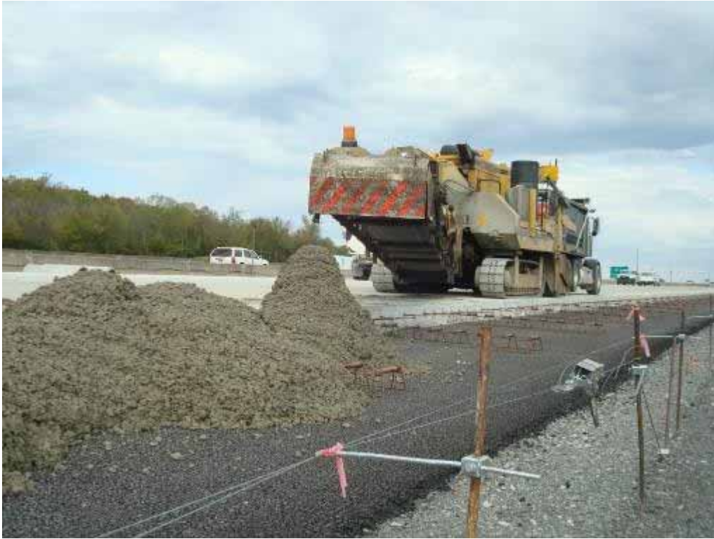
Photo E-13. Bottom lift concrete deposited on base by belt placer ahead of paver.
