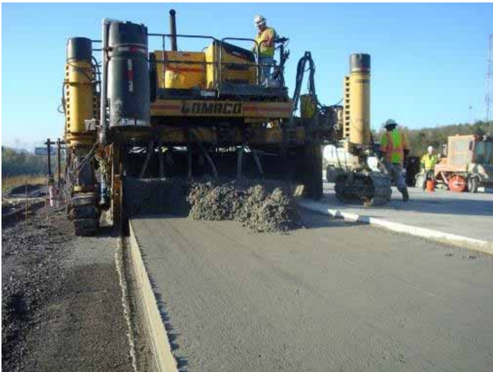
Photo E-42. Day 2 top lift placement, viewed from in front of paver.
