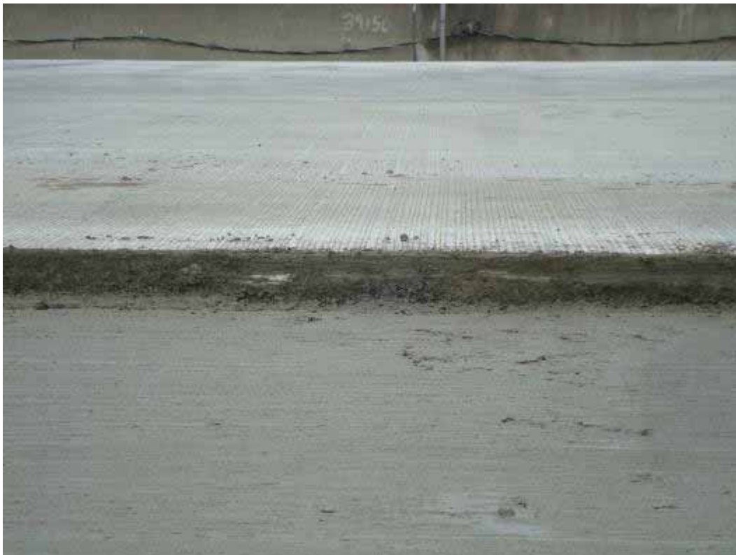
Photo E-20. Bottom lift surface behind paver (note: top lift will need to be more than 3 inches thick in this area).
