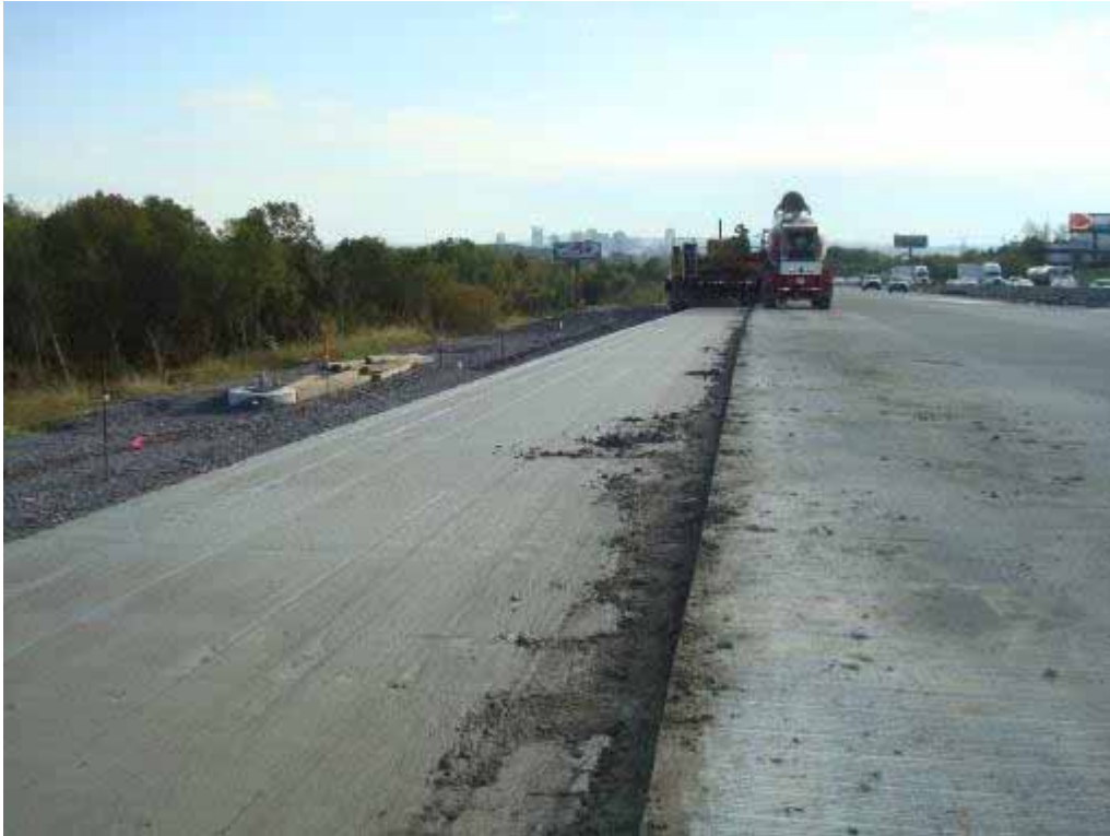
Photo E-25. Dowel “shadowing” in bottom lift surface and surface condition ahead of top lift placement at end of Day 1.
