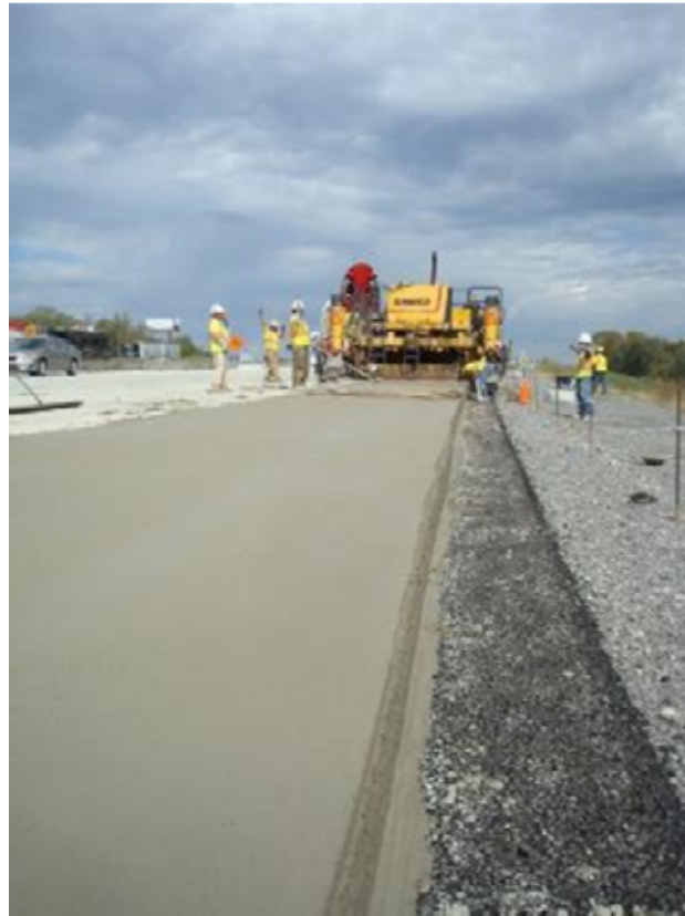
Photo E-29. Shoulder edge line after first edge slump correction effort.
