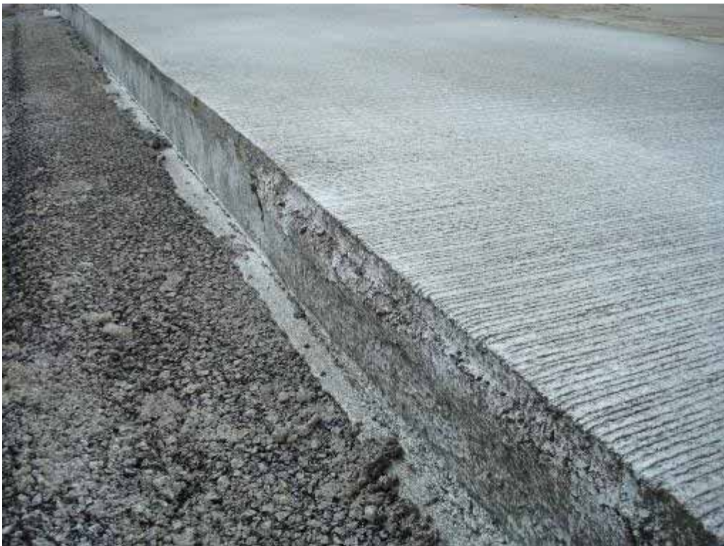
Photo E-32. Edge blowout #2.
