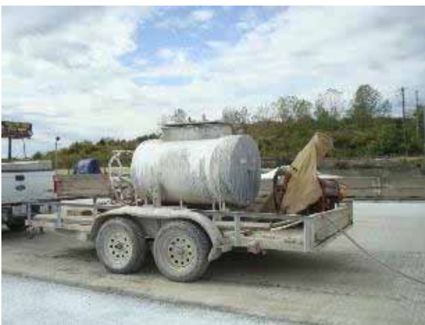
a. Curing compound storage tank.
