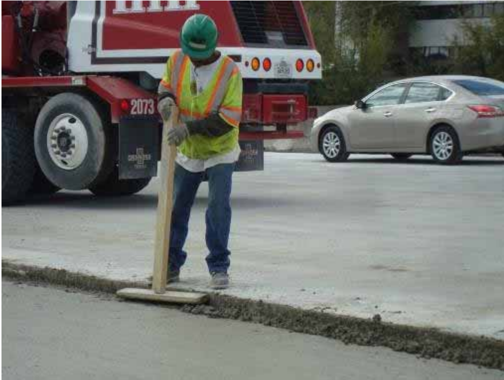
Photo E-21. Worker tamping down excess concrete at lane/shoulder joint after placement of bottom lift.
