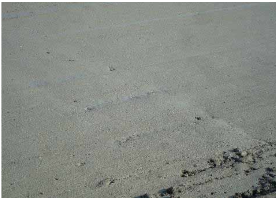
Figure 14. Thin bottom lift with dowel bar “shadowing.”
