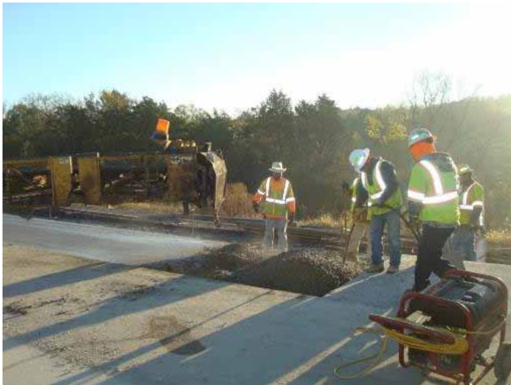
Photo E-40. Hand placement to close gap with header at start of Day 2 paving.
