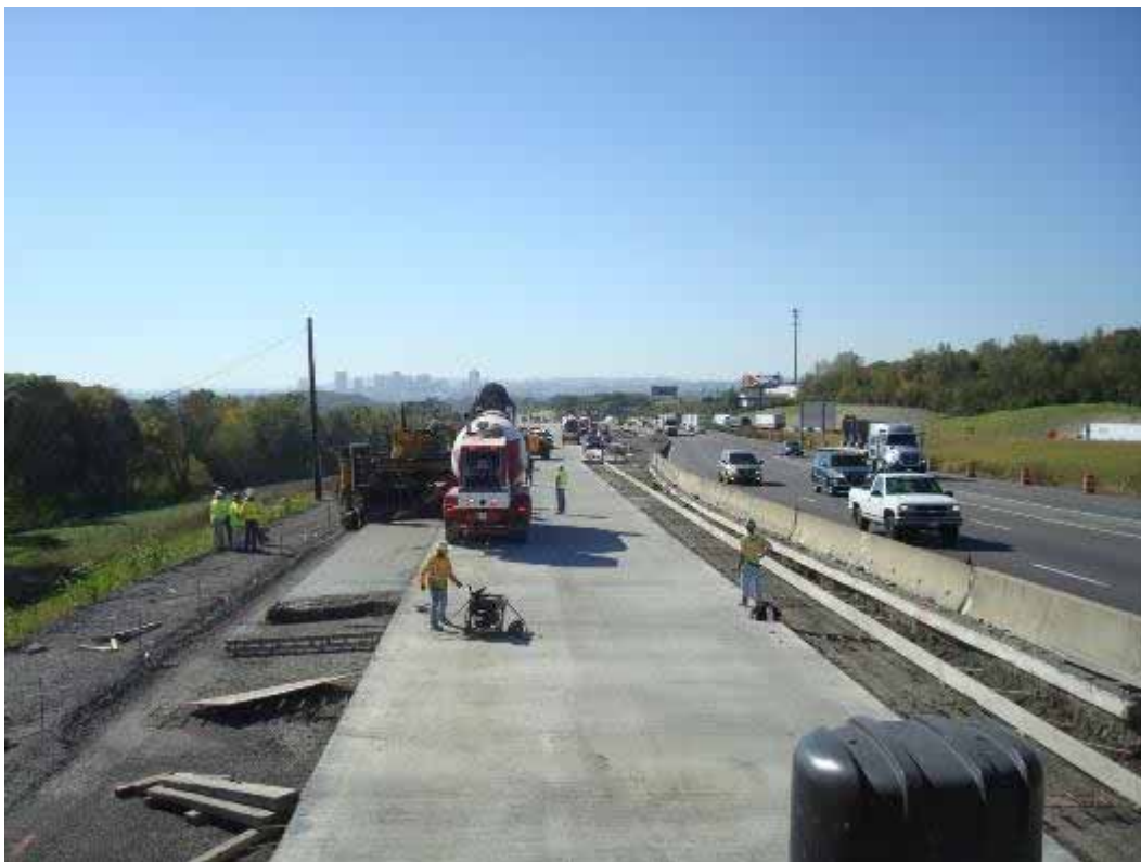
Photo E-2. North end of project looking south near end of Day 2 paving operations.
