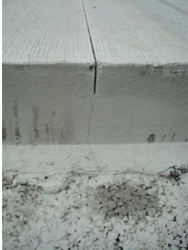
Photo E-57. Activated transverse joint in two-lift pavement.
