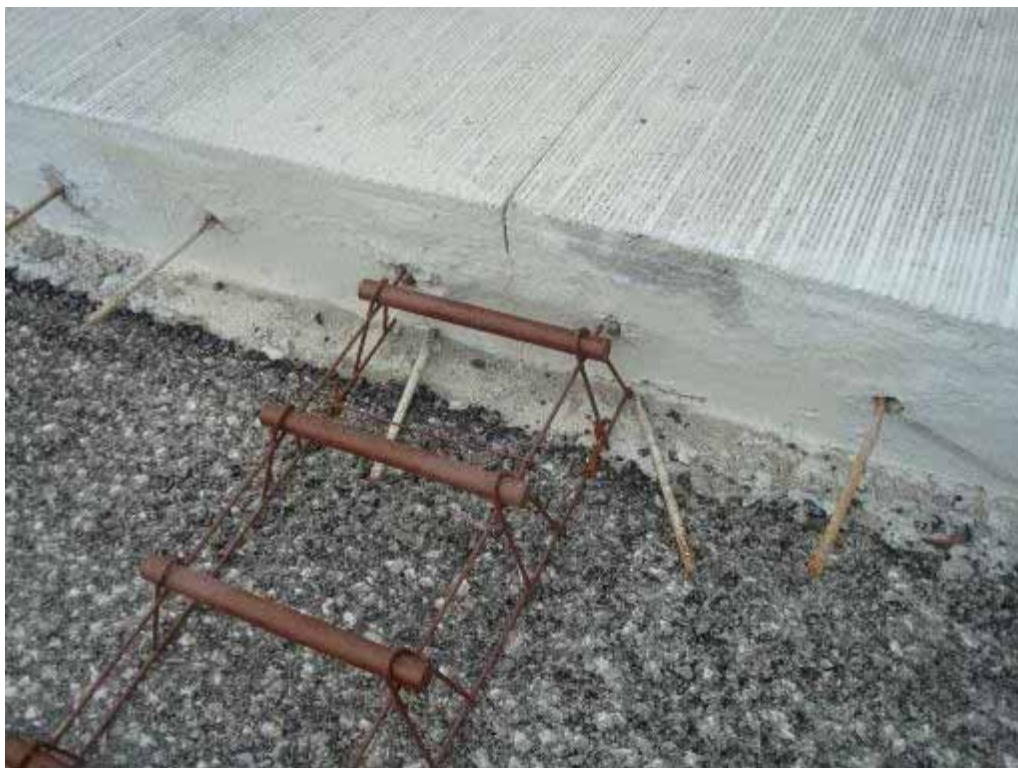
Photo E-4. Dowel basket placement showing proximity to travel lane and interfering with tie bars.
