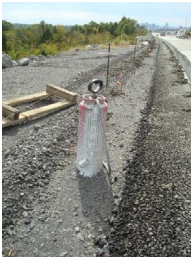
Photo E-54. "Garden sprayer" used for applying cure compound to outside shoulder edge.
