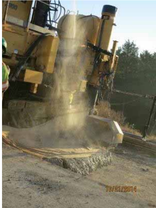
Photo E-39. Water being sprayed on burlap drag at start of Day 2 placement.
