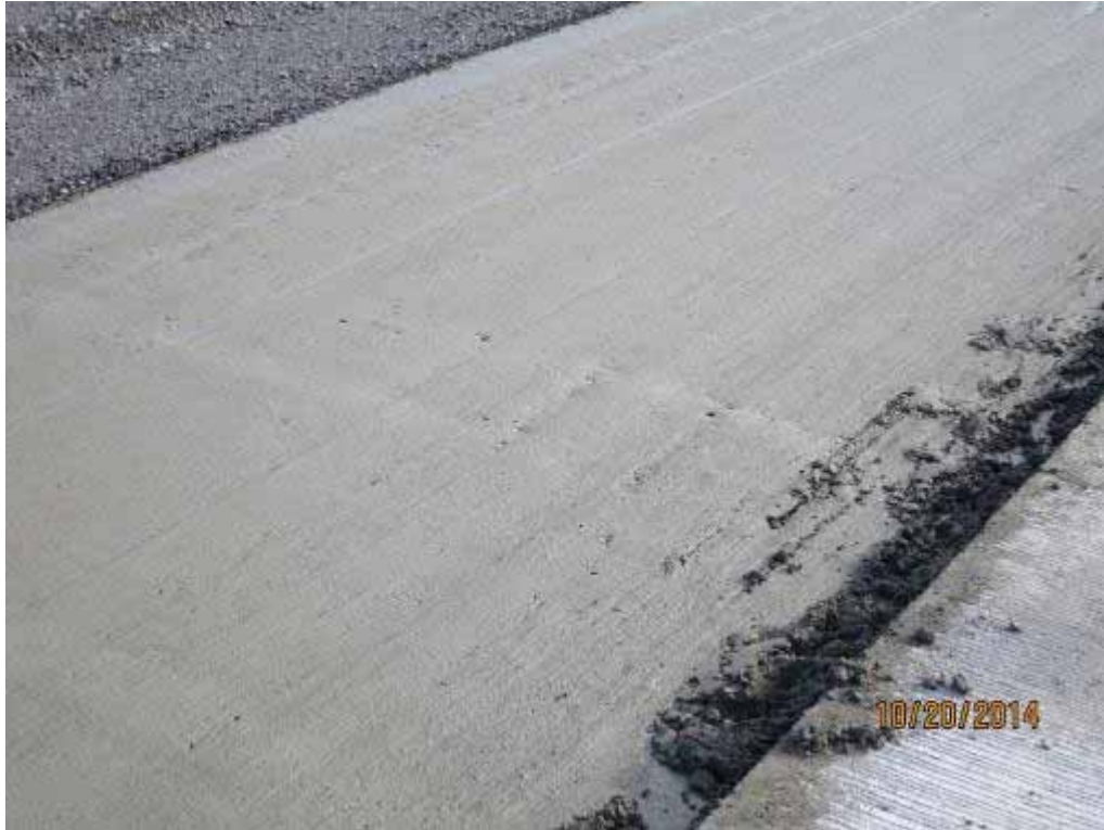
Photo E-23. Dowel “shadowing” and surface depressions and debris near end of Day 1 placement of bottom lift.
