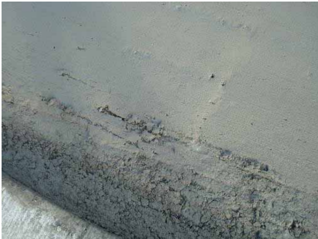
Photo E-24. Exposed dowel end in bottom lift due to thin lift.
