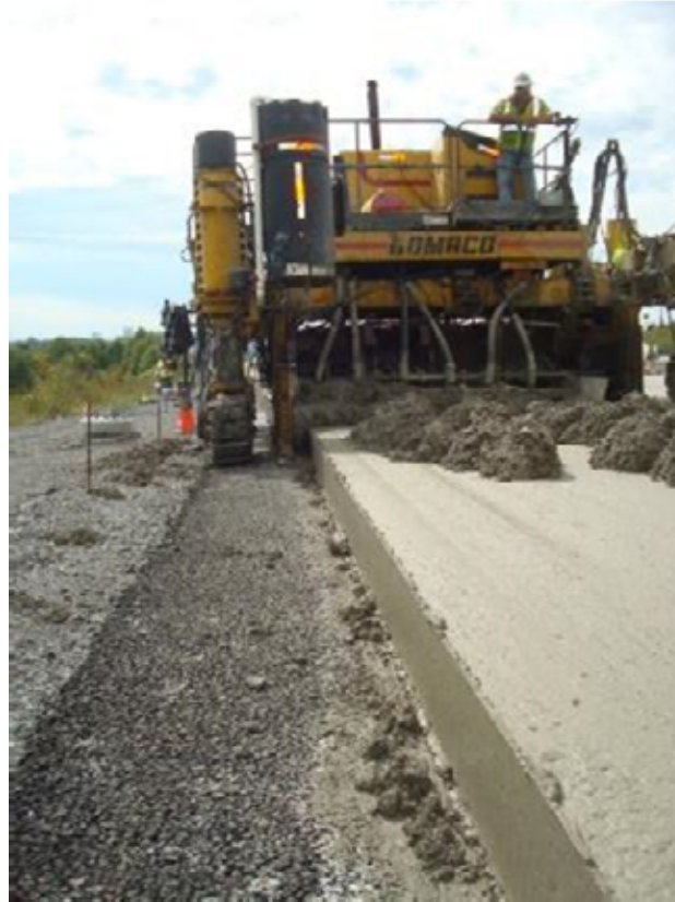
Photo E-27. View of top lift paving from in front of paver.
