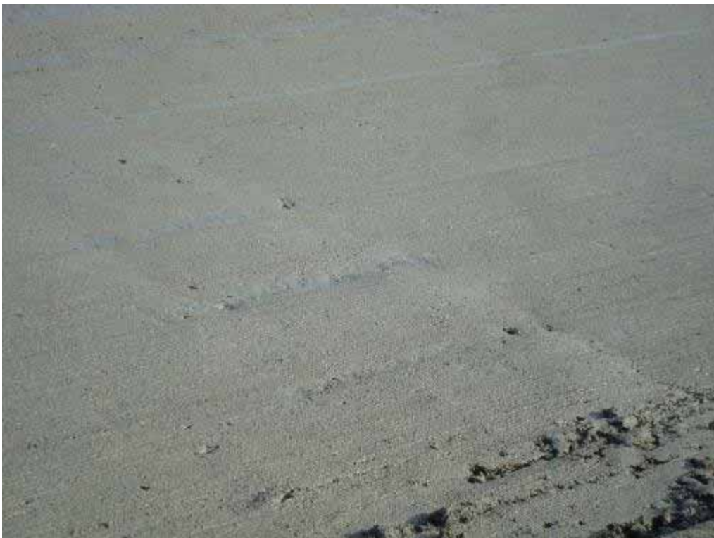
Photo E-22. Bottom lift surface “shadowing” due to proximity of dowels (thin lift).
