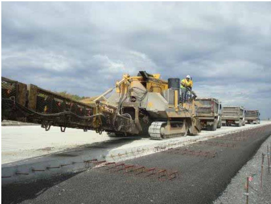
Photo E-12. Dump trucks and belt placer used for transport and placement of bottom lift concrete.
