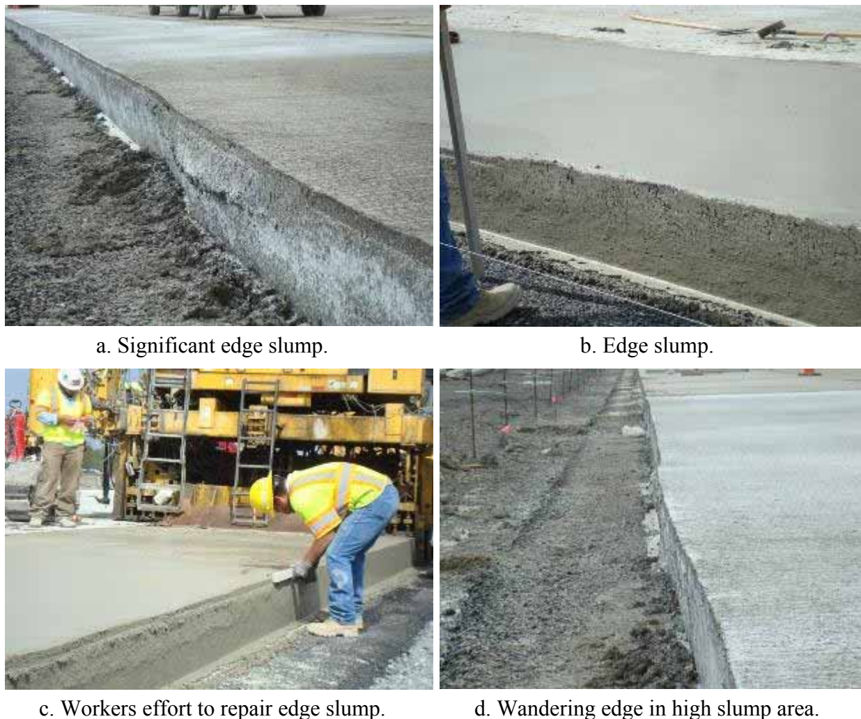
Figure 12. Edge slump and “blowouts.”
