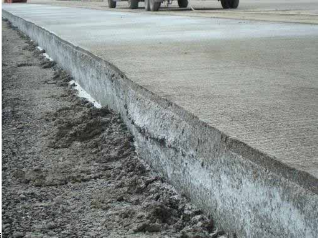
Photo E-31. Edge blowout #1.
