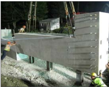
Rochester Fast 4, Bridge 16, setting abutments during weekend bridge closure. (Photo courtesy VTrans.)
