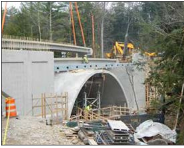
Middlebury Sand Hill Bridge, VT 125, recreating a historic arch structure with precast components. (Photo courtesy VTrans.)
