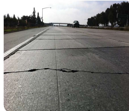
Faulting - Concrete Pavements
