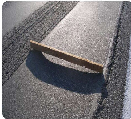
Rutting - Asphalt Pavements
