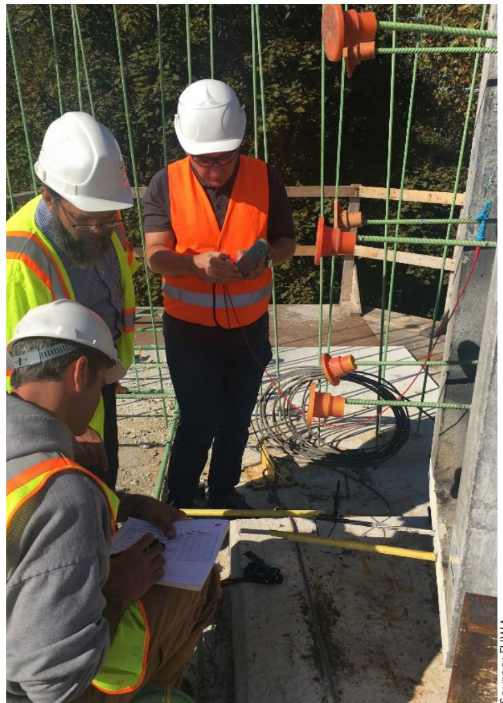
The main advantage of EIT systems is the ability to non-destructively monitor tendon encapsulation over time. In the photo above, initial construction reading is collected.
