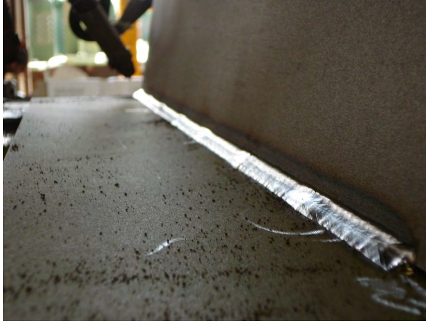
Figure 7-10 The Tack Welds Under this Cover Pass Were Re-melted, Yet Their Location is Still Obvious (This Condition is Acceptable because Profile Meets Code). The Larger Tack Welds Can Influence the Weld Profile
