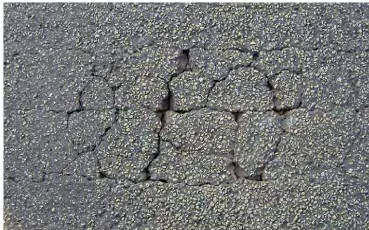
Figure 8-4 Visual Observations Indicating Deck Plate Crack as Evidenced by the Overlay Deterioration (de Jong, 2006)
