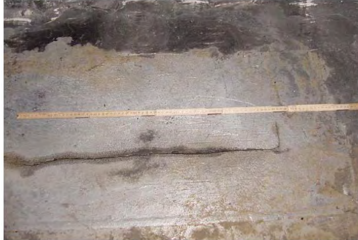
Figure 8-5 The Deck Plate Crack is Verified after Removal of Asphalt Layer (de Jong, 2006)
