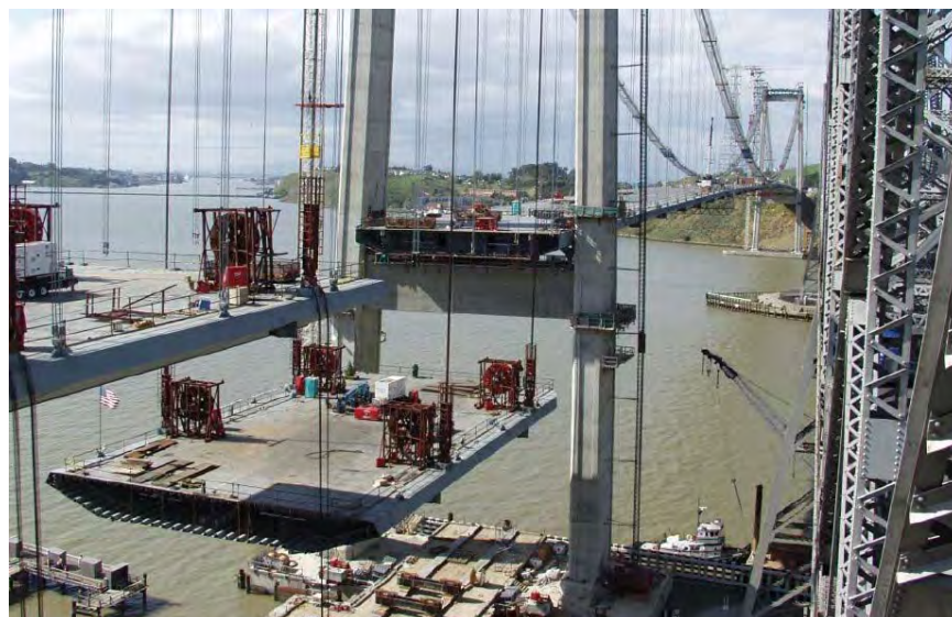
Figure 1-2 Erection of Orthotropic Box Girder Segment for the Alfred Zampa Memorial Bridge lifting a Deck Segment into Place
