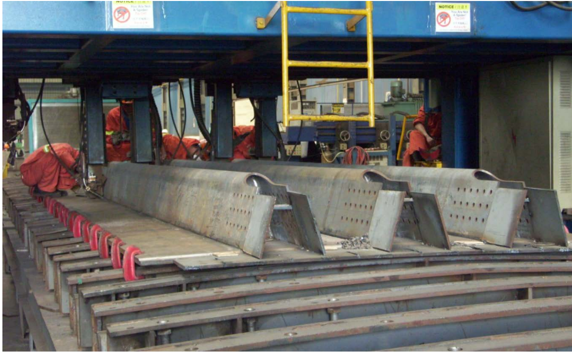
Figure 7-5 Fabricators Automate where Possible to Improve Productivity and Quality such as Using the Gantry as shown which Allows Three Ribs to be Welded at One Time
