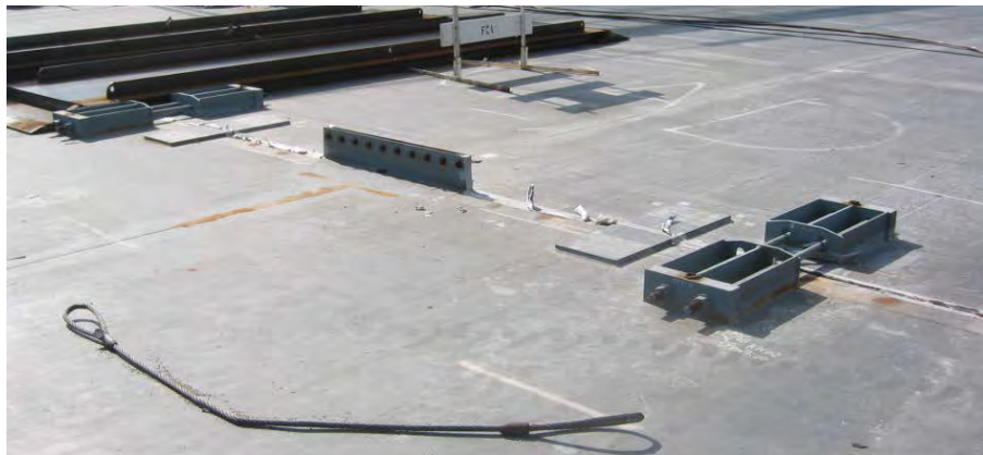
Figure 7-15 Temporary Fit-Up Lugs are Necessary for OD Construction. Tensioning Rods Bridge Two Sections to Pull Together and Align the Adjacent Panels
