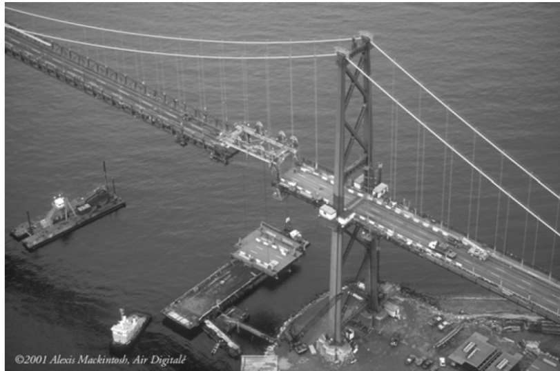
Figure 2-4 Aerial Photo of the Lions Gate Bridge showing the Redecking with Orthotropic Deck Segments being Lifted into Place
