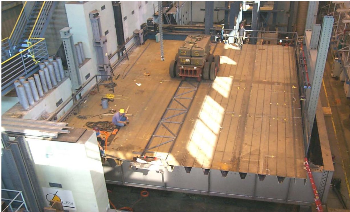
Figure 10-2 Test Setup for the Prototype of the Bronx Whitestone Bridge Redecking Tested at Lehigh University showing the Deck, Loading Truck, and Loading Guide
