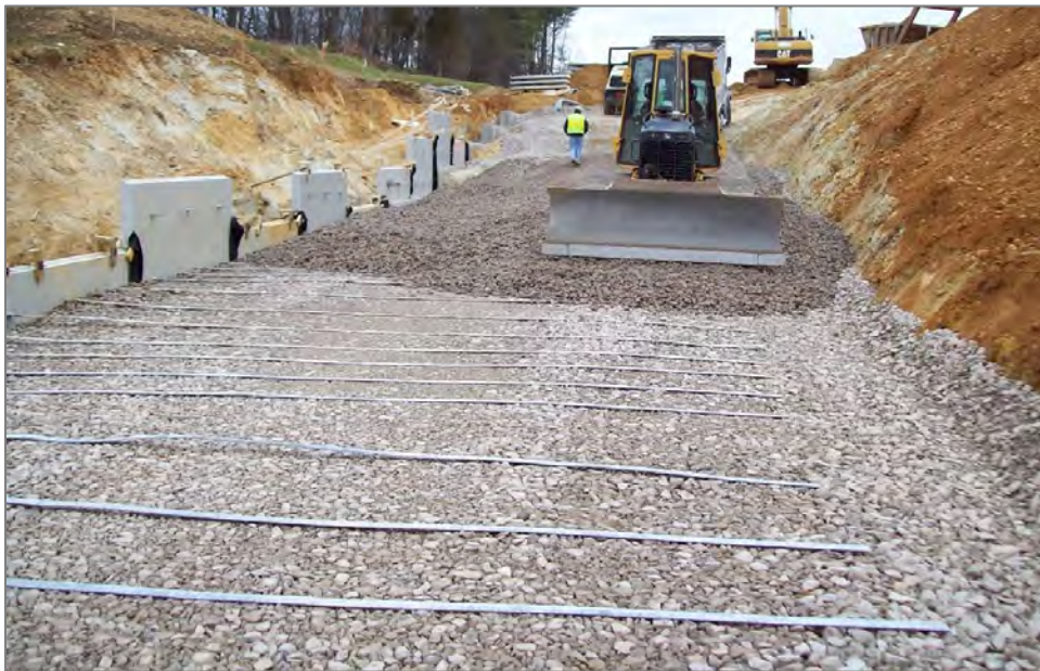
Figure 28: Placement of the reinforced fill over the first layer of reinforcing elements
