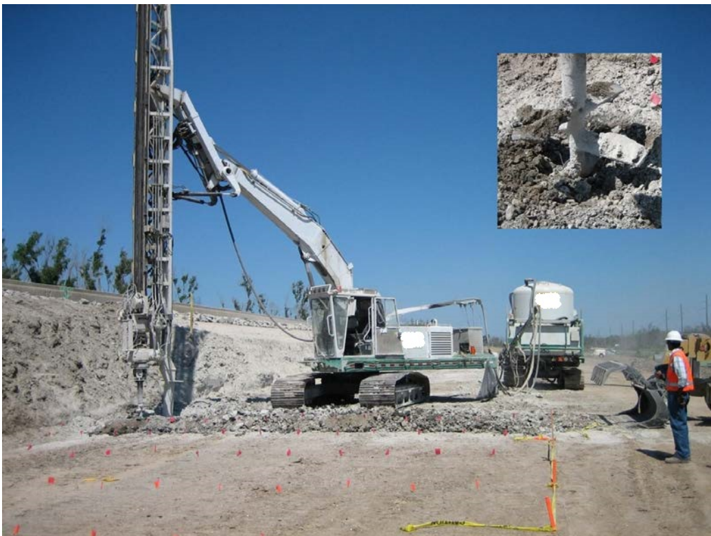
Figure 7-2. Deep mixing by the dry method; insert shows blades of mixing tool, with port for binder delivery on shaft.
