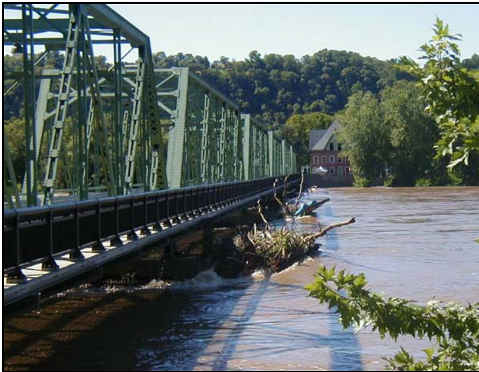
Figure 3.12. An example of debris blockage on piers.
