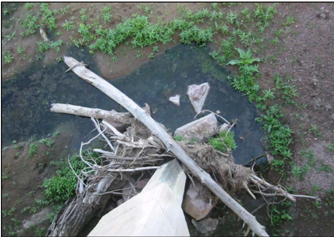
Figure 8.7. View down at debris and scour hole at upstream end of pier.
