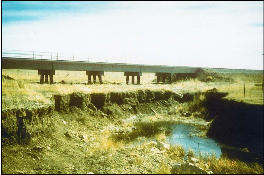
Figure 8.10. Headcut downstream of a bridge.
