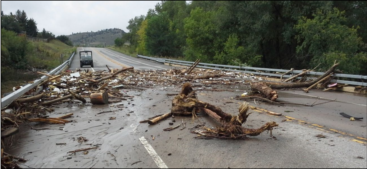
Figure 6.8. Flood debris on a bridge deck.
