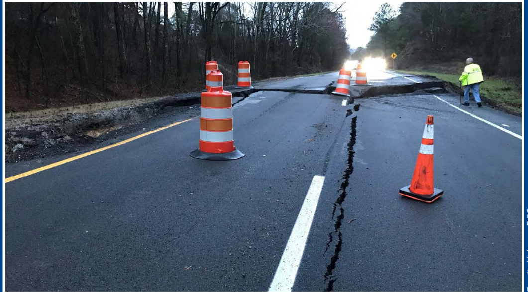
Initial slope movement closing US-231 due to massive landslide in Lacey's Springs, Alabama.
