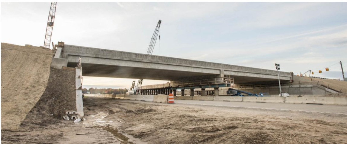
Figure 8 - Elevation of Bridge after Slide
