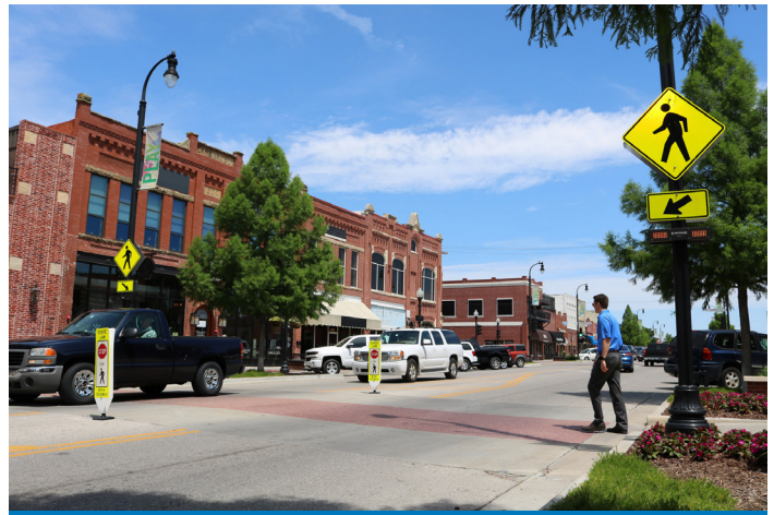
The city of Broken Arrow installed a passive pedestrian-activated RRFB in the Rose District (above).
