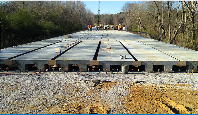
The South Carolina Department of Transportation evaluated the use of three types of beams with UHPC connections on a Kershaw County bridge project.
