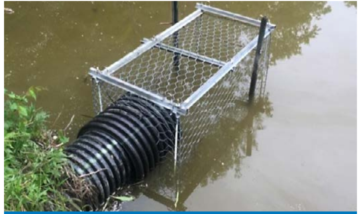
The beaver pipe cage keeps the animals from packing culverts with sticks and mud.
