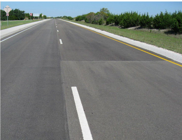
Advanced, proven preservation practices can help extend the overall service life of pavements.
