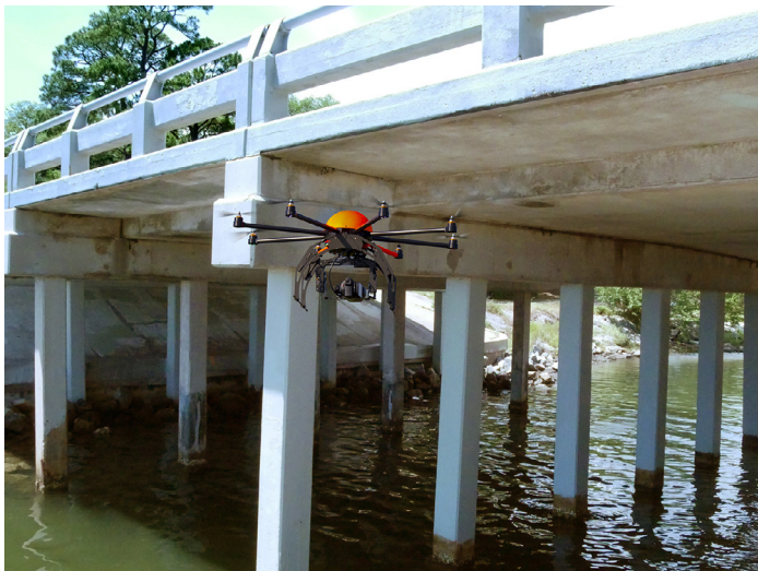
UAS can support traditional bridge inspection practices to provide rapid, high-quality data.
