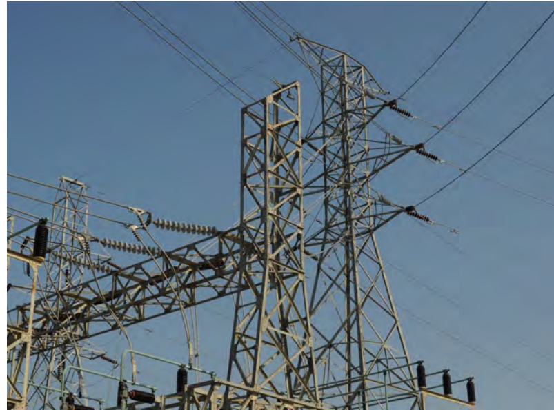
ODOT consolidated over 3,000 various electric and gas utility accounts. - Ohio Department of Transportation
