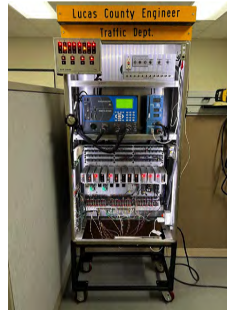
Equipped traffic signal ready to analyze defective equipment - Lucas County Engineer's Office
