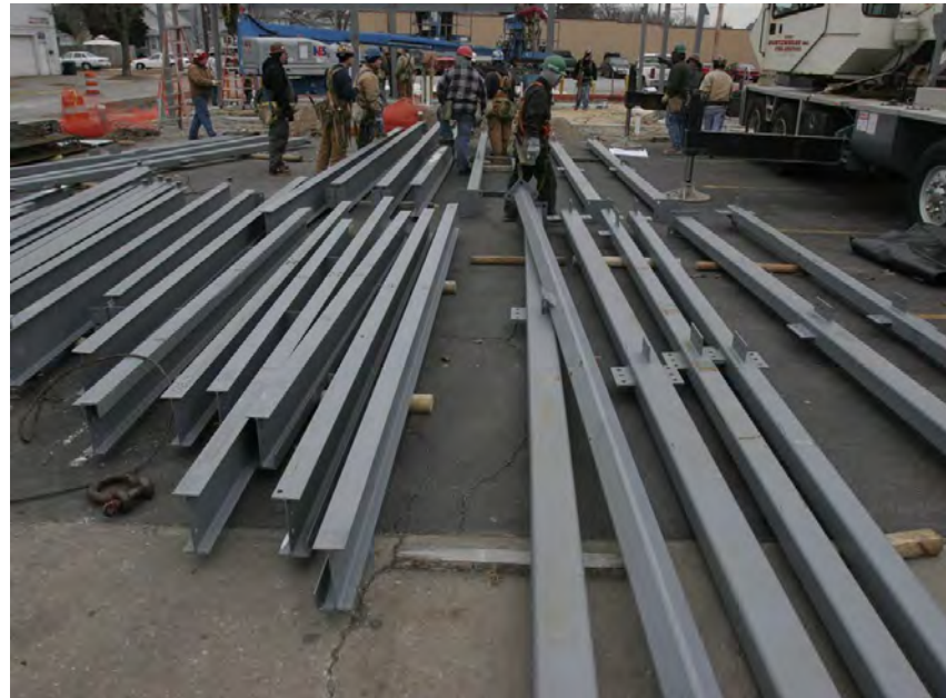
Upcycled bridge beams ready for a local construction project. - The Toledo Blade newspaper
