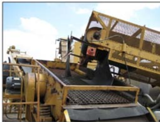
Figure 21. Photo. Smaller scalping screen for large RAP particles.
