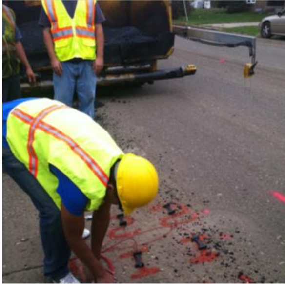
Figure 164. Photo. Installation of the prototype packaging system installed during a construction project near Lansing, MI.
