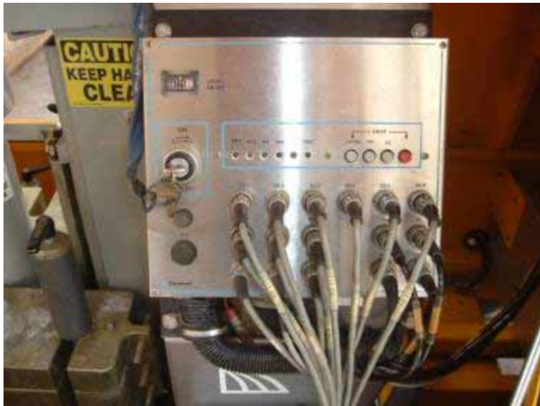
Figure 135. Power control box (board behind front panel).
