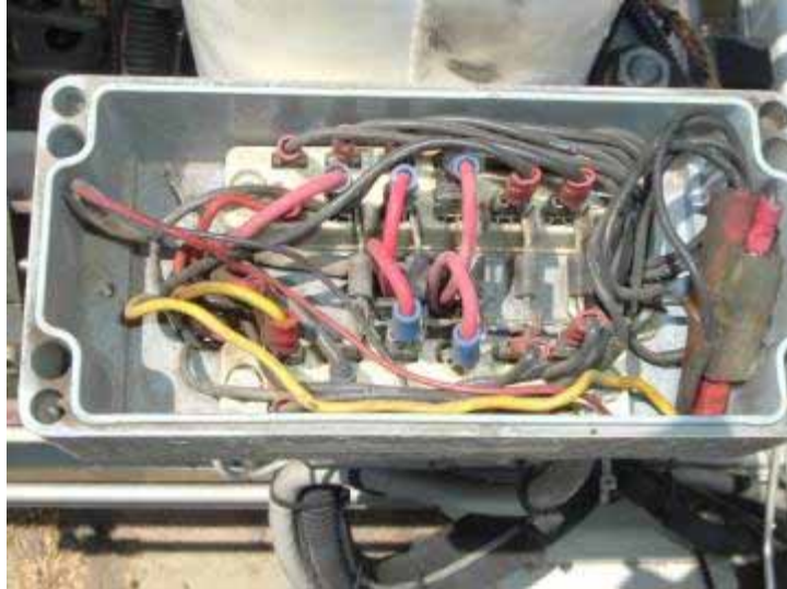
Figure 129. Electronics connection box.
