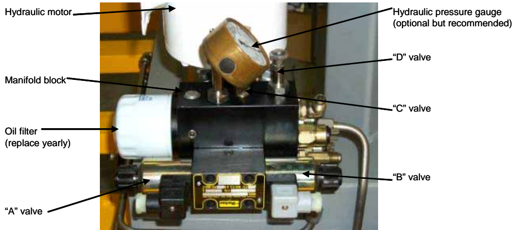
Figure 44. Manifold block and A/B valve mounted to hydraulic pump.
