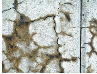
Figure 2. Closeup view of cracking on concrete barrier along State Route 2 near Leominster, MA.
