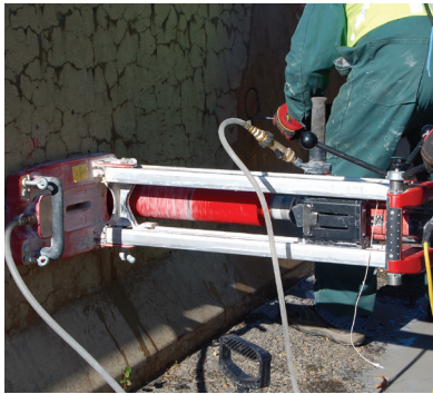
Figure 3. Coring equipment being used to extract a 10-centimeter (4-inch) diameter core from a concrete barrier.
