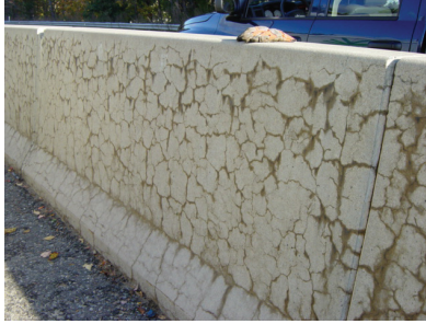
Figure 1. Extensive map cracking in several concrete barriers along State Highway 2 near Leominster, MA.
