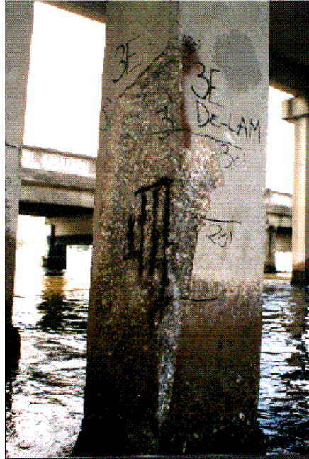
Figure 1. Photograph of a cracked and spalled marine bridge piling.
