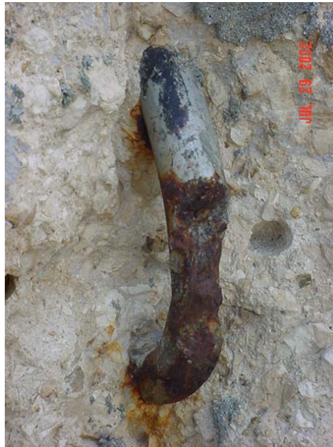
Figure 25. Corrosion of an exposed reinforcing bar.
