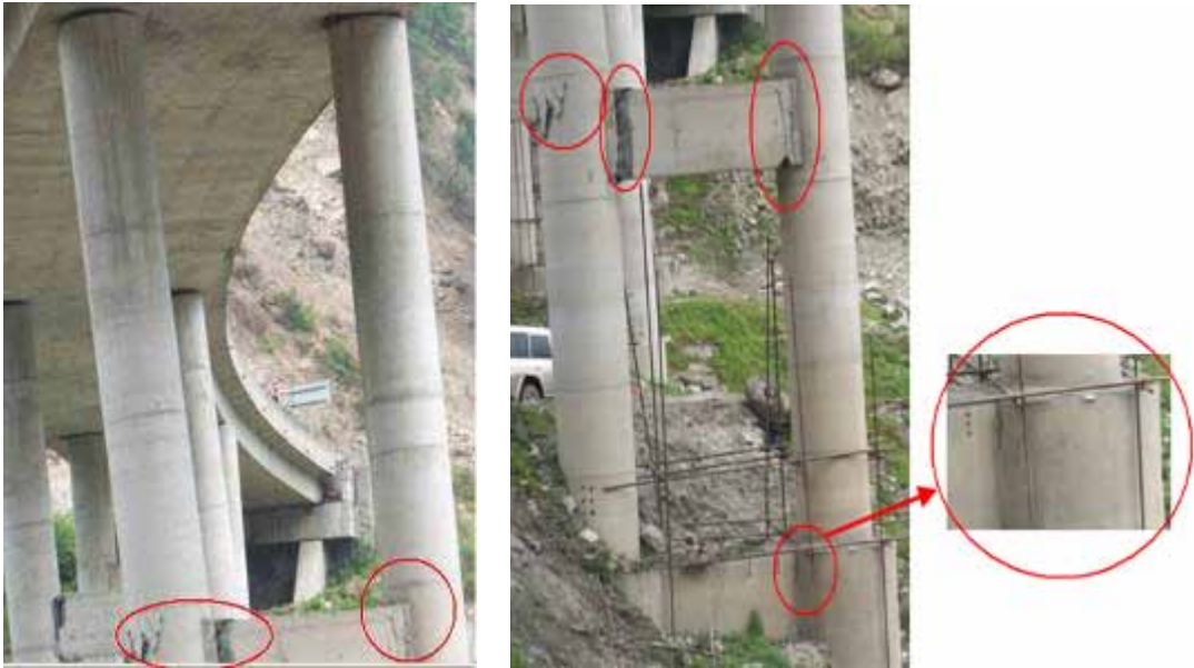
Figure 65. Photo. Damage at Bent 3.
