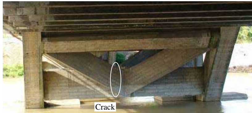
Figure 26. Photo. Cracks on Diagonal Members/Transverse Bracings.
