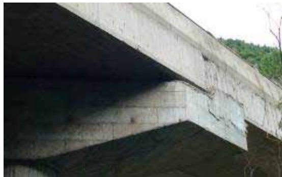
Figure 31. Photo. Damage in Shear Key.
