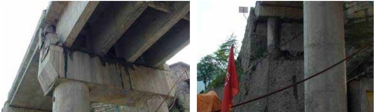
Figure 59. Photo. Damage to Shear Key and Embankment of the Overpass.
