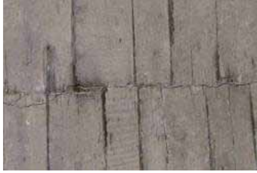
Figure 39. Photo. Transverse Crack at the Crown of Secondary Arch.
