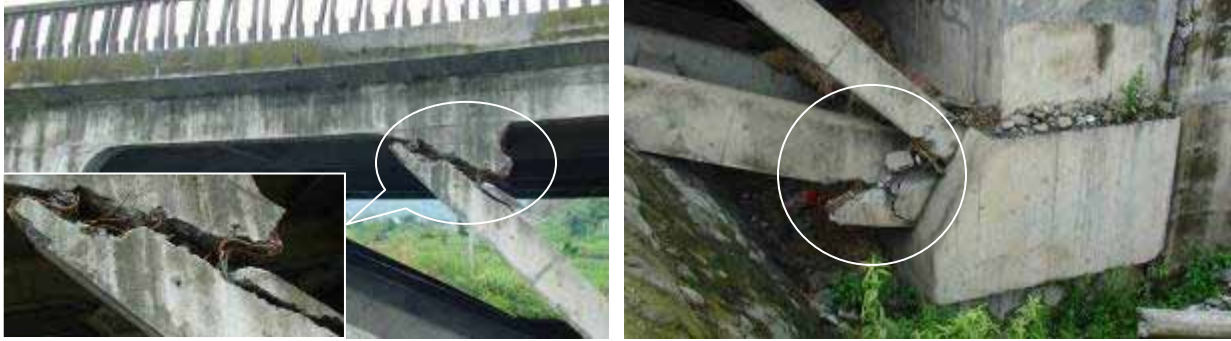
Figure 20. Photo. Details of Shear Failures in Easternmost Span.
