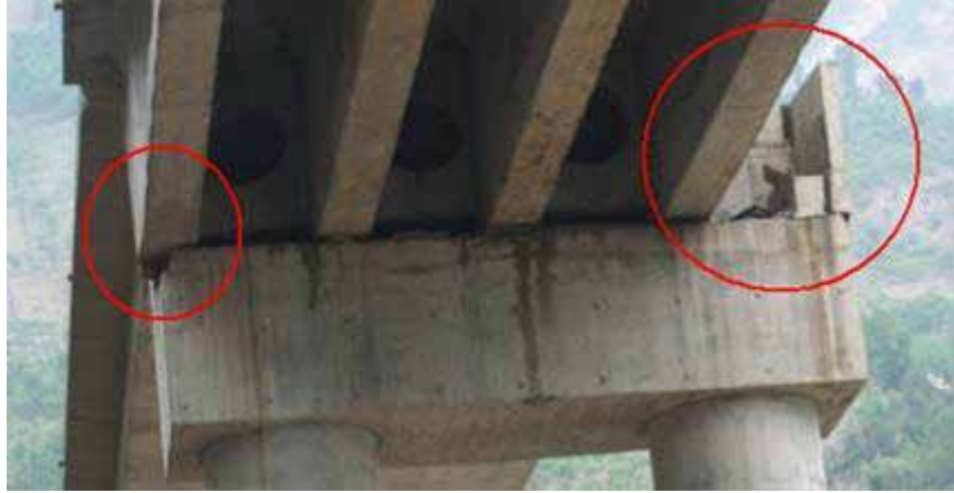
Figure 66. Photo. Damage at Bent 9.
