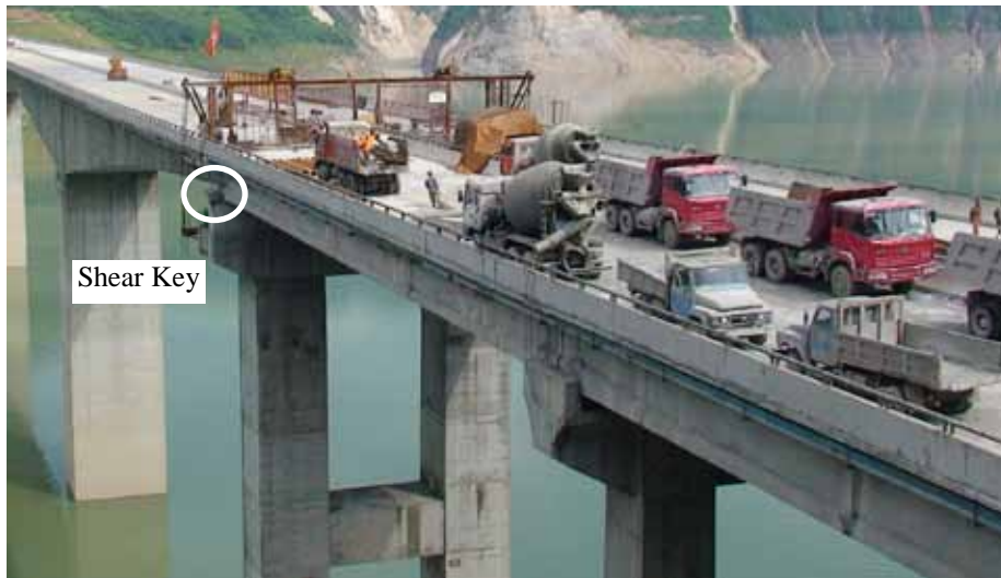
Figure 57. Photo. Shear Key Failure.
