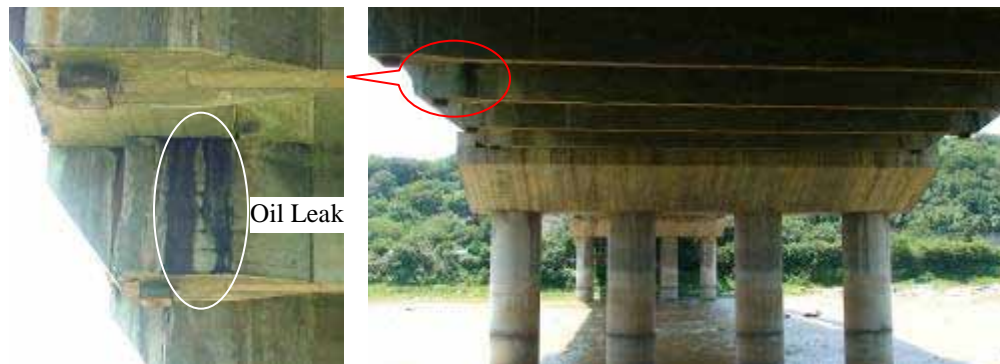
Figure 36. Photo. Oil Leakage Underneath the Bridge Deck.
