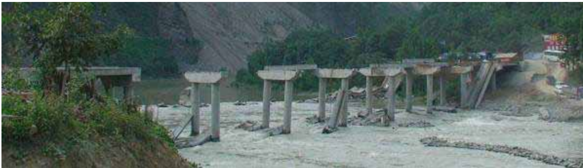
Figure 47. Photo. Damage Scenario of 10-Span Bridge Under Construction During the Earthquake.
