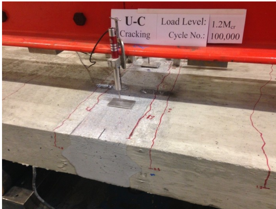
Figure 166. Photo. Observed cracking in specimen U-C after pre-cracking cyclic loading.
