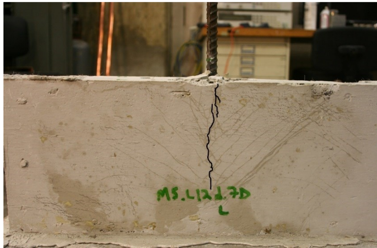
Figure 142. Photo. Bond test failure due to side splitting.
