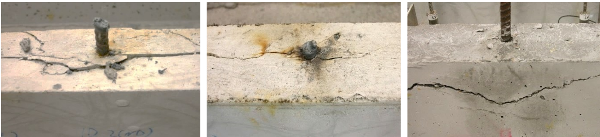
A. Wide splitting cracks: U-D with V_f = 1.5 percent B. Thin splitting cracks: U-D with V_f = 2.5 percent C. Cone failure: U-C with V_f = 4.5 percent
