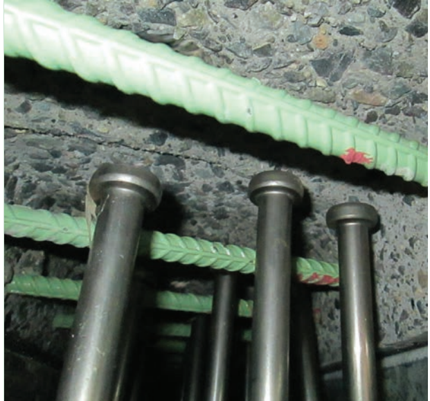
Figure 25. Photo. Hidden pocket connection detail with shear studs extending above the bottom mat of rebar to allow use with non-UHPC grouts or concretes. (25)
