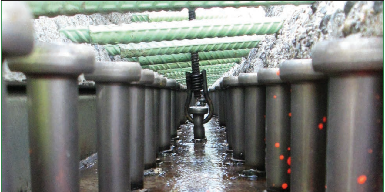
Figure 23. Photo. Longitudinal connection detail above first interior girder line with shear studs stopping below the bottom mat of rebar. (25)
