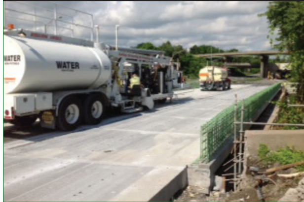
Figure 17. Photo. Surface profiling of a bridge deck on I-690 near Syracuse, NY.
