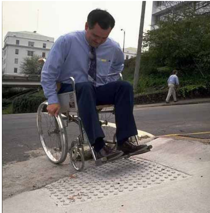
Figure 8-18. Photo. A pavement grinding project left an exaggerated lip at this curb cut.
