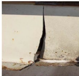
Condition State 4 (Cracking/Fatigue)
