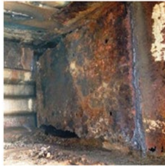
Condition State 4 (Corrosion)
