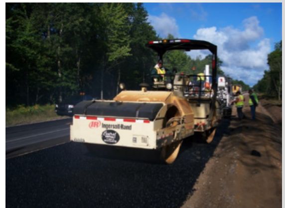
The use of performance contracting on the M-115 rehabilitation project enabled the contractor to offer a five-year pavement warranty.
