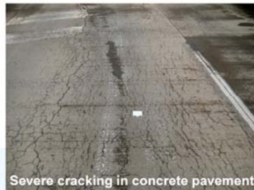
Severe cracking in concrete pavement
