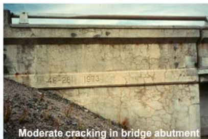
Moderate cracking in bridge abutment
