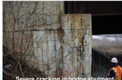
Severe cracking in bridge abutment
