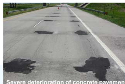
Severe deterioration of concrete pavement
