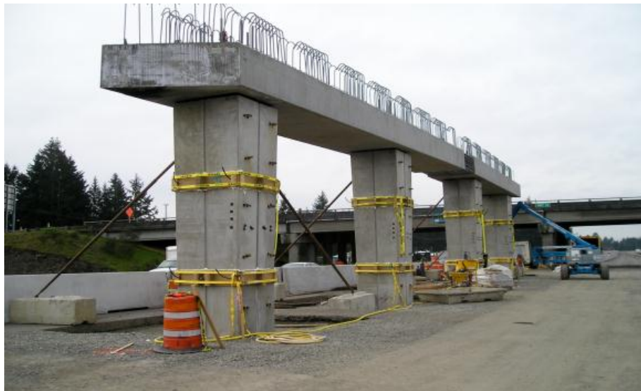
Figure 48. Photo. Grouting the joints between column segments and between columns and cap beam.
