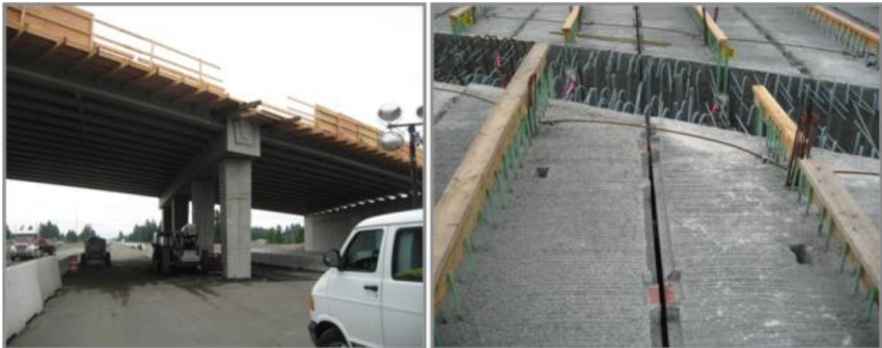
Figure 49. Photo. Placement of precast girders and preparation for deck slab topping concrete.
