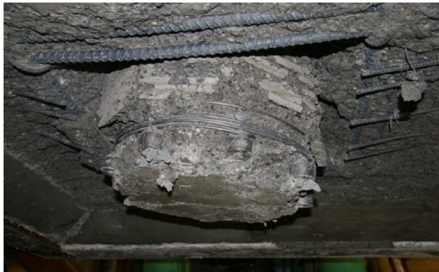
Figure 28. Photo. Specimen SF-3 footing failure.
