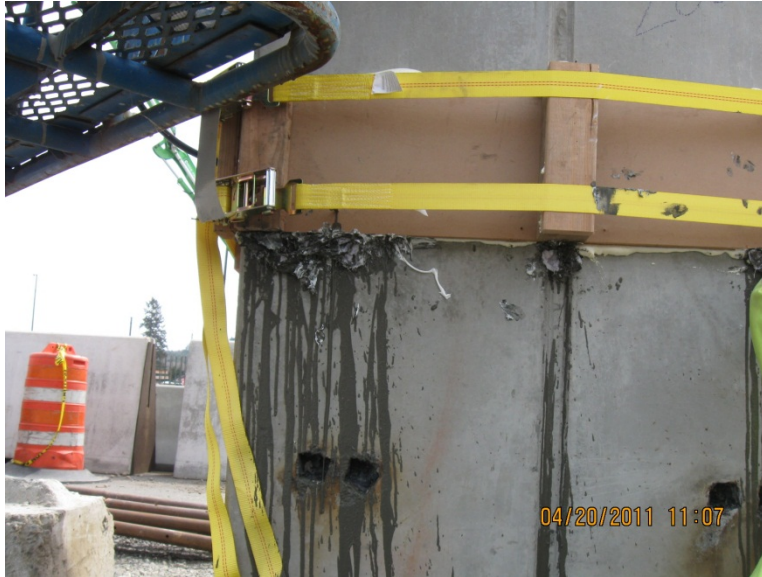
Figure 52. Photo. Difficulty with sealing the column segment joint during grouting.
