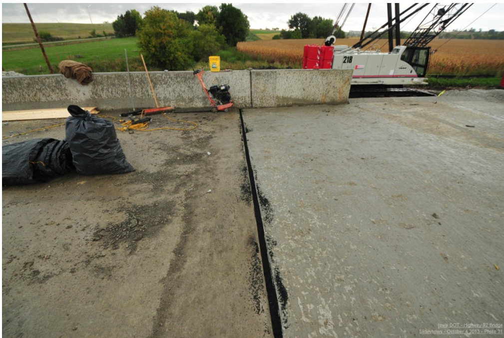
Figure 38. Photo. Expansion joint (courtesy: Iowa DOT).
