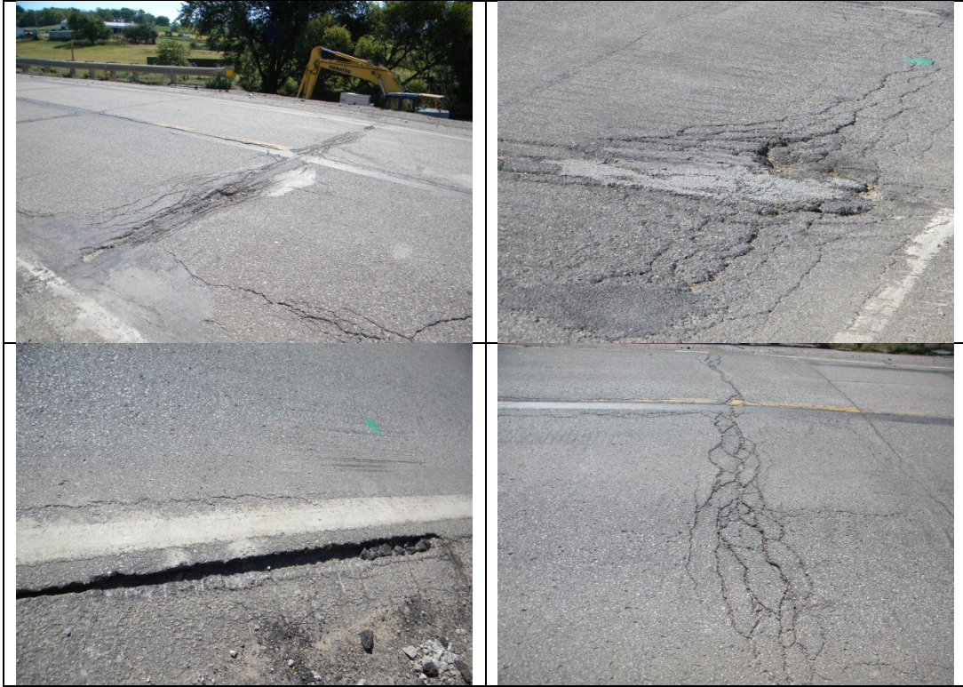
Figure 2. Existing Bridge Deck and Approach Roadway Conditions
