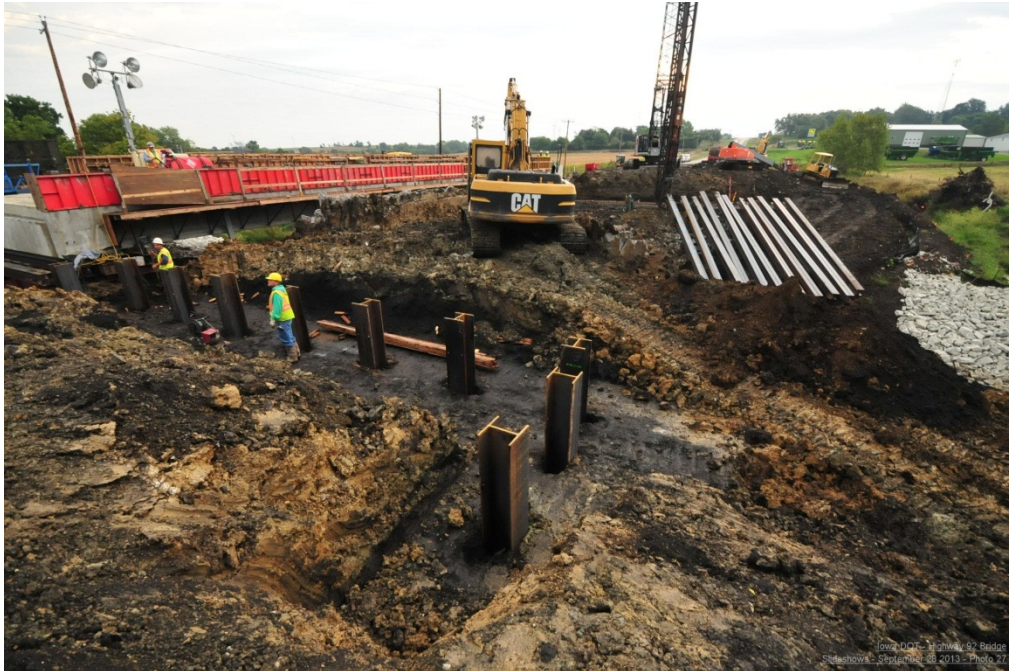
Figure 17. Photo. HP 14x117 (courtesy: Iowa DOT).
