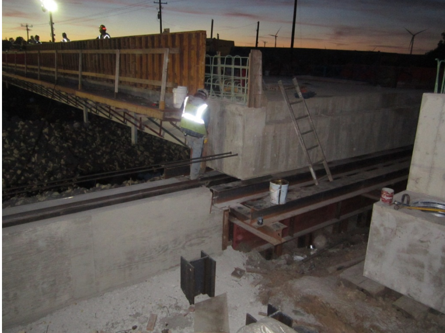
Figure 25. Photo. Start of slide (courtesy: Iowa DOT).
