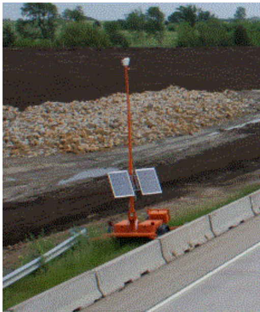
Figure 6. Photo. Noncontact sensor used to collect traffic data.
