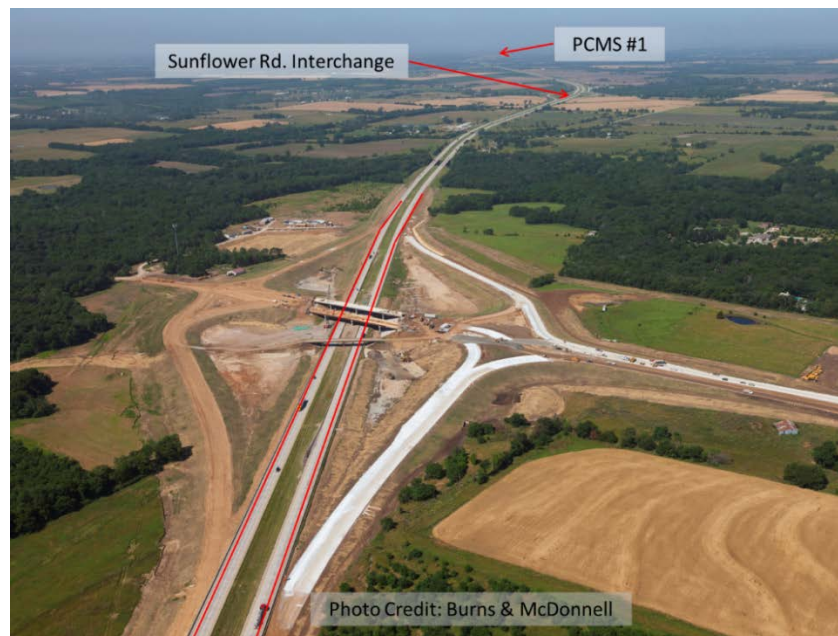
Figure 2. Photo. First portable changeable message sign location. (courtesy: KDOT)
