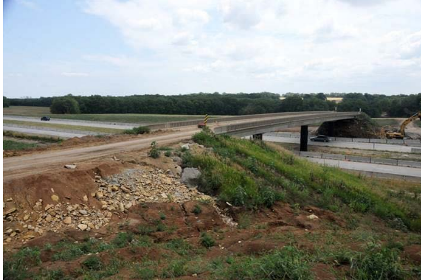
Figure 3. Photo. Homestead Lane Bridge over I-35 being demolished during an overnight closure. (courtesy: KDOT)
