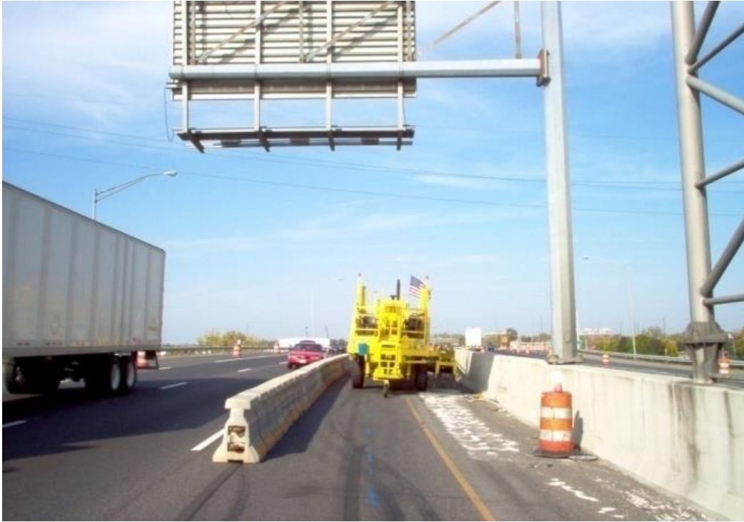
Figure 27. Photo. Movable barriers providing access at ramps.
