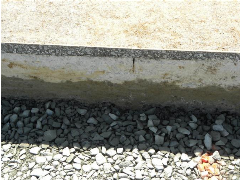
Figure 14. Photos. Joint sawing and AC surfacing over a sawcut in the RCC layer
