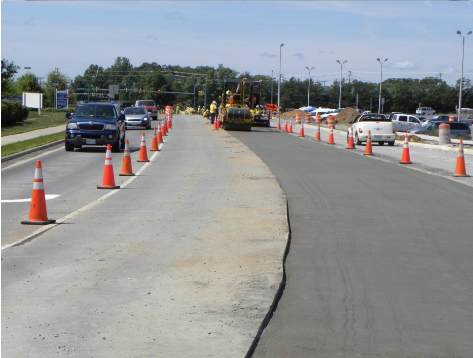
Figure 11. Photos. RCC compaction behind the paver (with rollers operated in a static mode).
