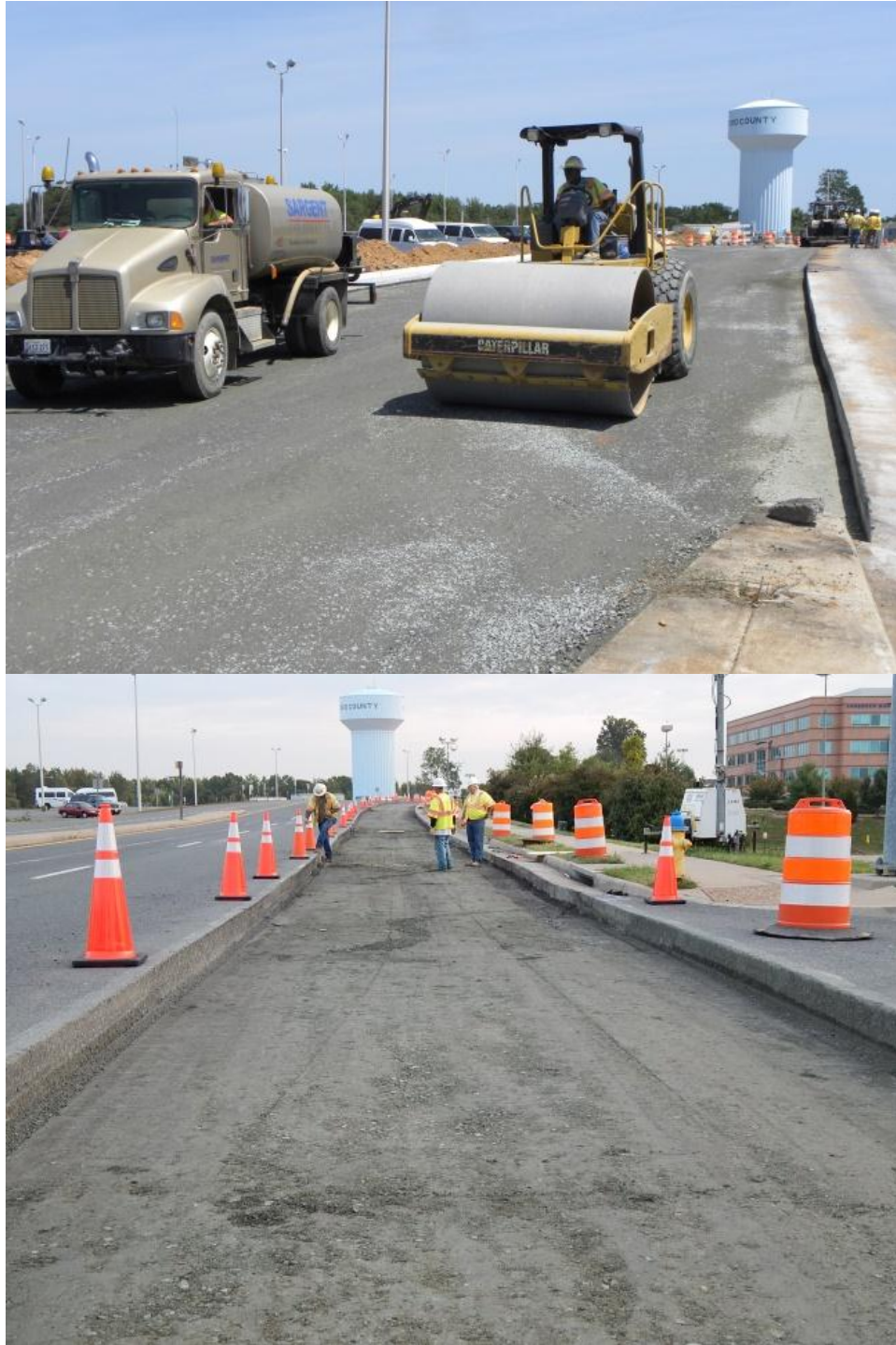
Figure 7. Photos. Base compaction and finished base just before RCC placement. Note that geogrid was used to stabilize the subgrade prior to placement of the base.
