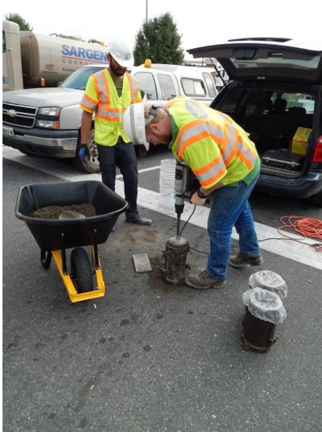
Top - Density testing using a nuclear gage, Bottom - Molding strength specimen Figure 12. Photos. Field testing during RCC placement.
