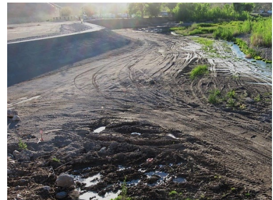
Figure 5: Gabion-lined training dikes upstream of the replacement Beaver Dam Wash Bridge. Source: Mohave County
