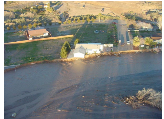
Figure 2: Damaged house and flooded bank on Beaver Dam Wash from 2005 flood. Source: Mohave County
