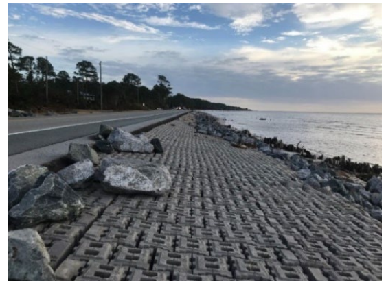
Figure 3: An Articulated Concrete Block (ACB) revetment system on US 98 in Florida. Source: FHWA
