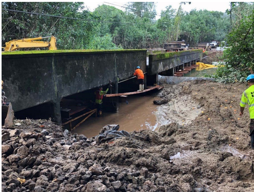
Figure 1: Side view of the historic Waipā Bridge illustrating the damage caused by the historic rainfall event in April 2018. Source: HDOT
