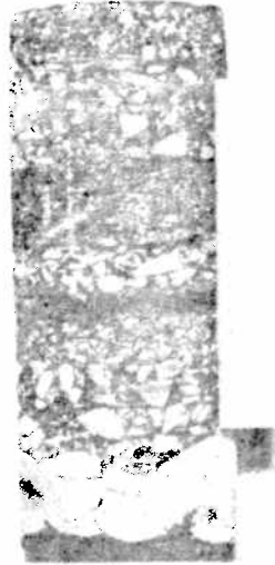
Figure 2. Core showing typical number of overlays on concrete base.
