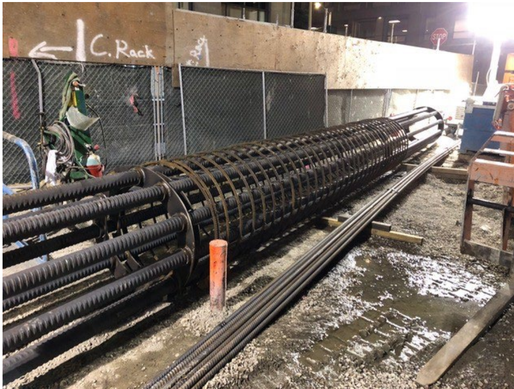
Figure 5-5 Reinforcing cage with Grade 75 threaded bars used for structural enhancement of a drilled shaft in which deficient concrete had been removed from inside the reinforcing cage.
