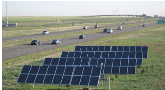
E-470 solar array.
