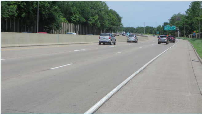
Category #0. No apparent distress. Candidate for monitoring to identify initial and progression of distresses.
