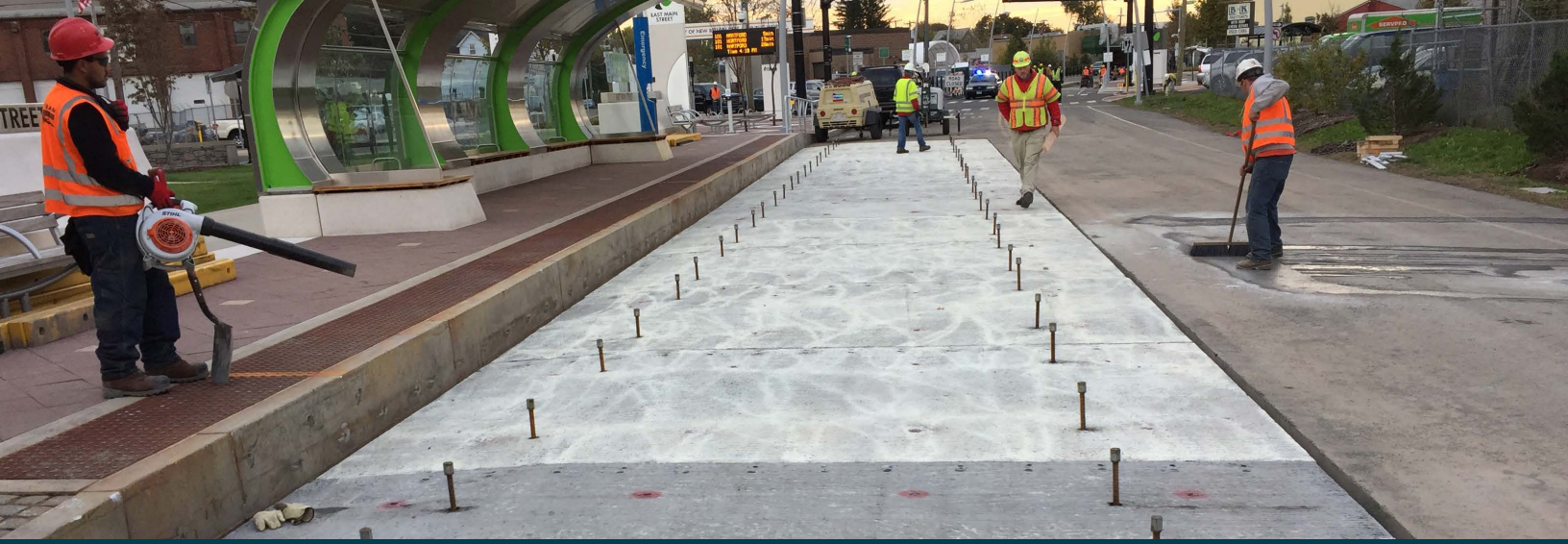
In Connecticut, PCP panels with leveling bolts engaged replaced a rutted asphalt bus pad. Source: FHWA.
