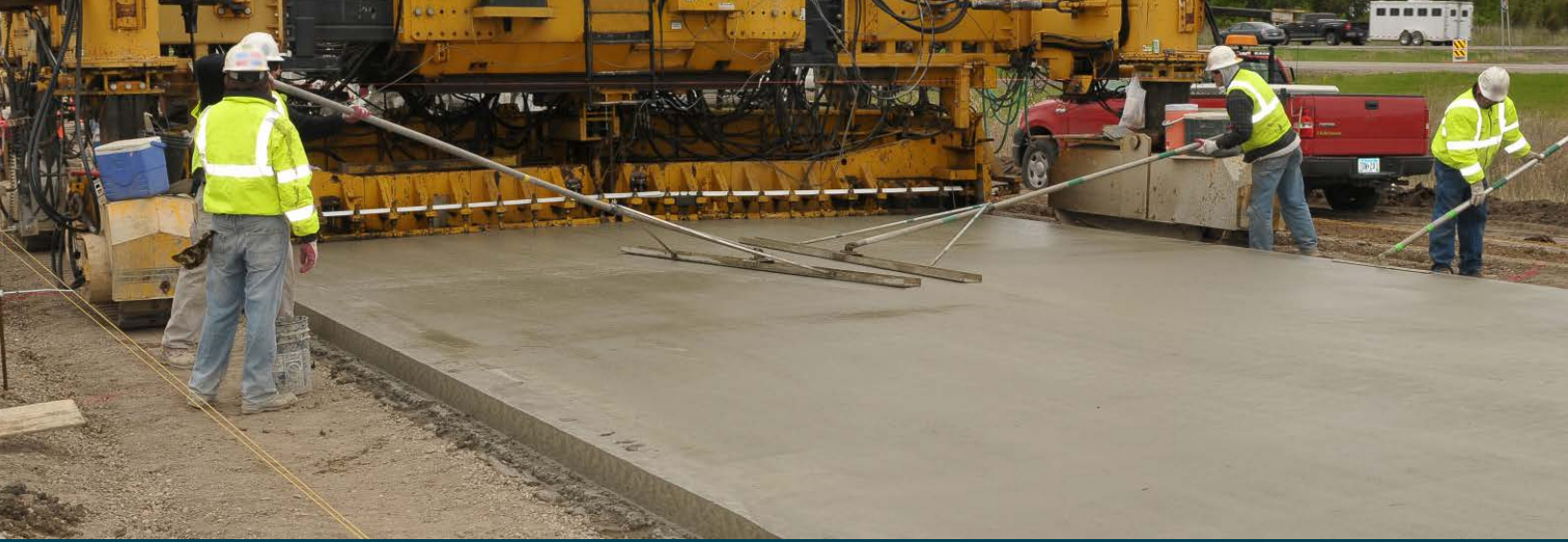
A construction crew is using a slipform paver to spread, consolidate, and screed concrete. FHWA recently published a Pavement Design Best Practices Catalog with recommendations related to pavement structures for both asphalt concrete and jointed plain concrete pavements. Photo: ©Shreenath Rao, Applied Research Associates, Inc.
