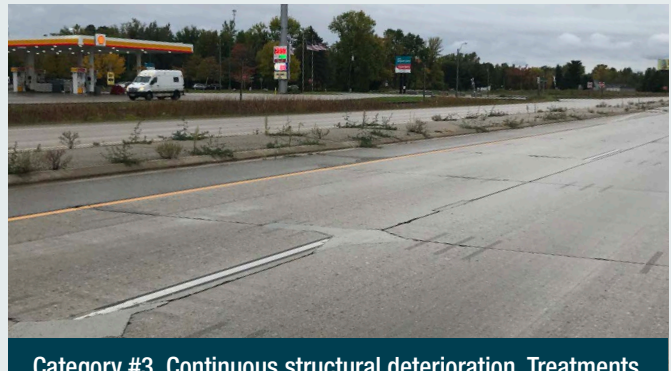
Category #3. Continuous structural deterioration. Treatments applied to maintain serviceability until major rehab or reconstruction can be performed.
