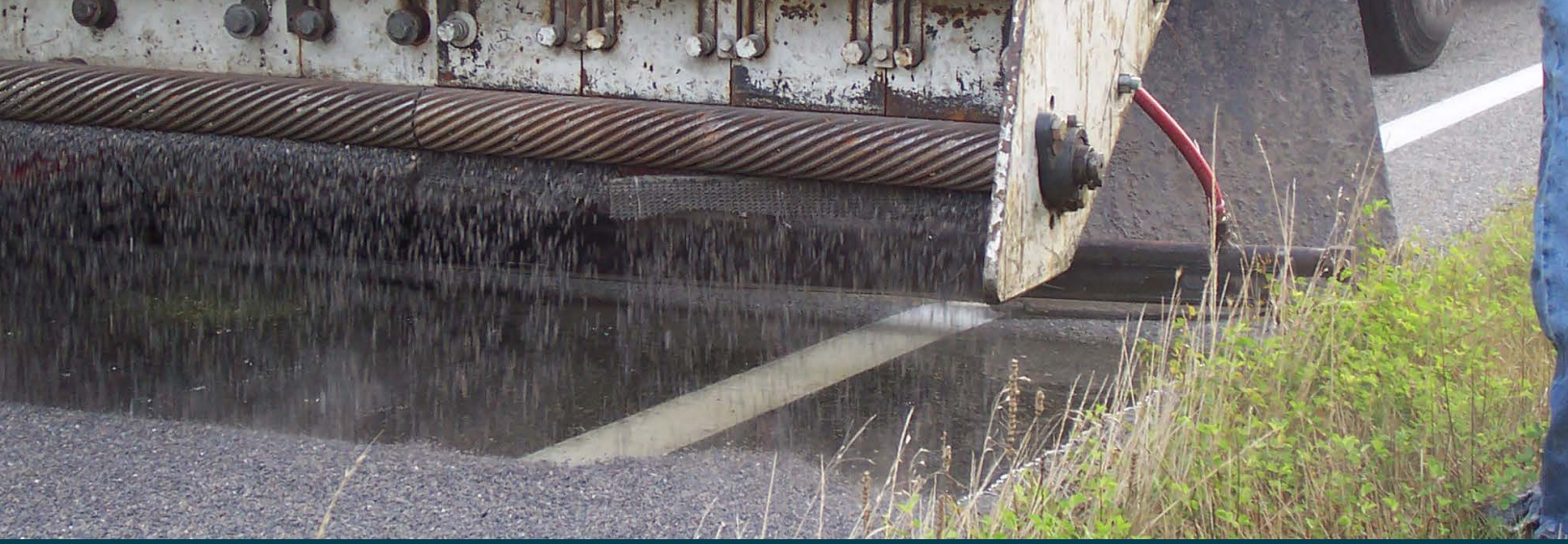
This aggregate spreader is using automated application to increase pavement friction on this road. Source: FHWA.
