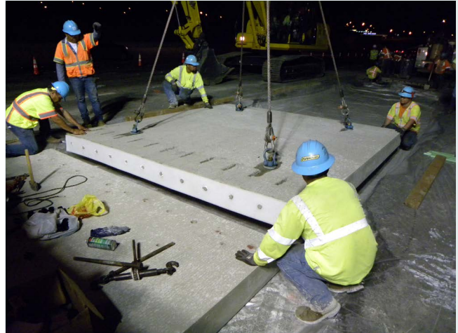
A construction crew lowers a PCP panel onto a prepared base as part of reconstruction of Interstate H-1 west of Honolulu, HI. Source: FHWA.
