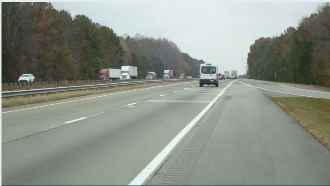
Category #2. Improvements (e.g., structural overlays) have been performed to prevent/arrest structural deterioration.
